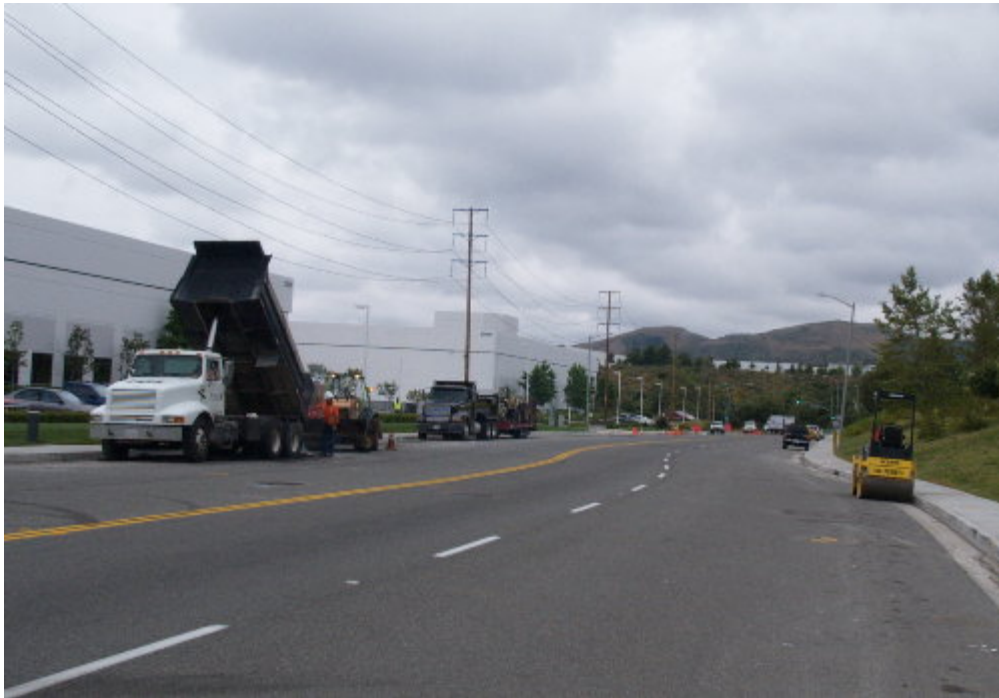
Figure 4 – Arizona Pipeline paved the trench-line and vault locations on Ellipse Road and across the intersection of Glenn Ranch Road.
