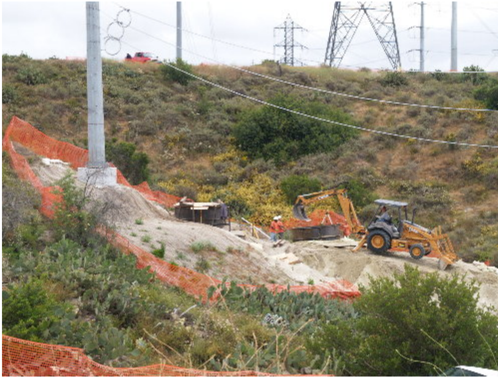
Figure 5 – The forms for the new foundations for Structure 13 were set during the site visit. The tops of the forms were covered for safety.
