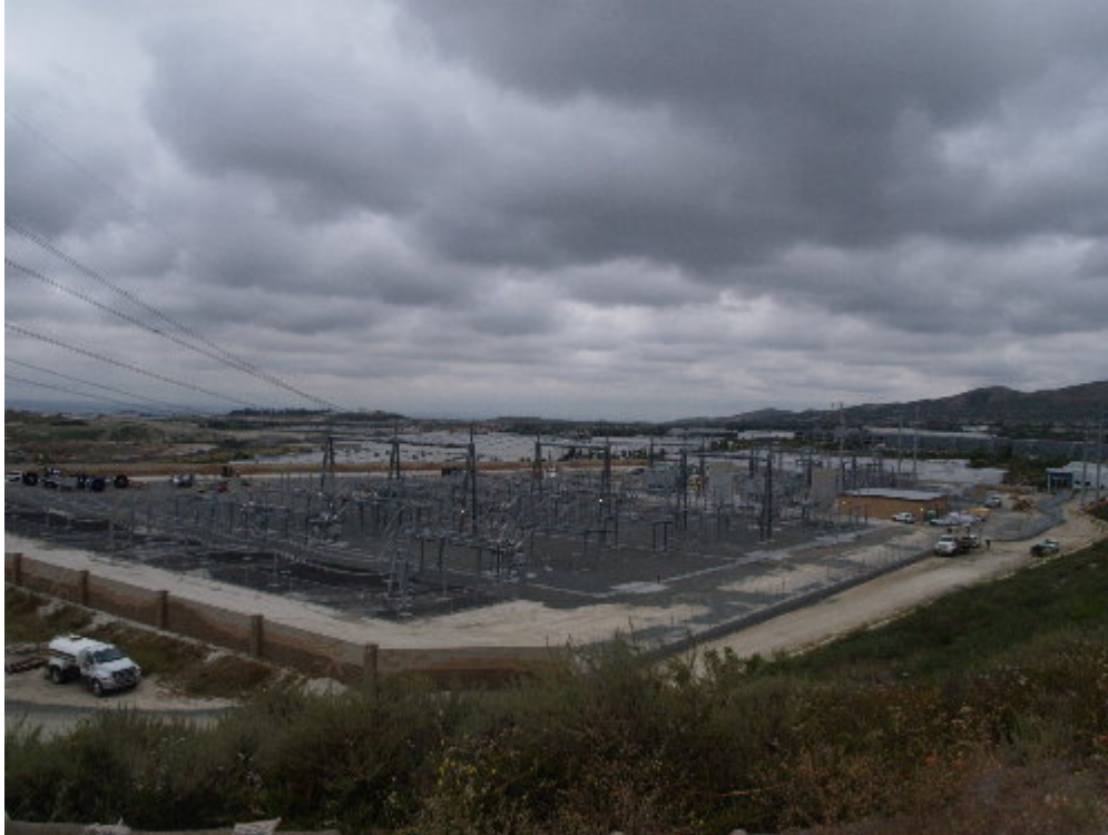
Figure 1 – Overview of the substation site after the 220 kV and 66 kV portions have been energized (66 kV section energized on May 31 st ).
