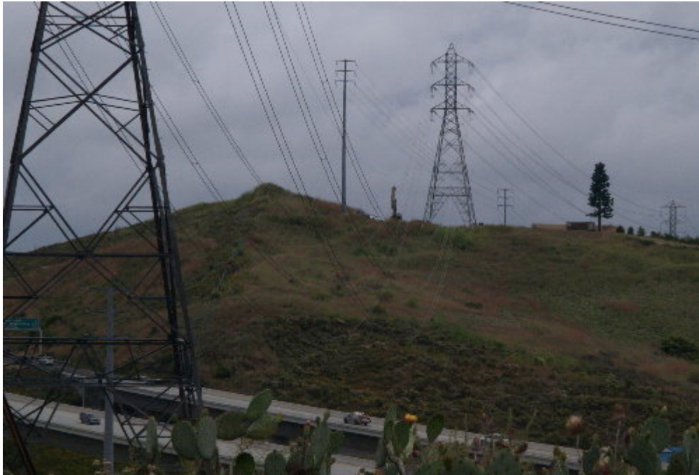
Figure 6 – Work started on the foundations for Structure 10, in the City of Mission Viejo.
