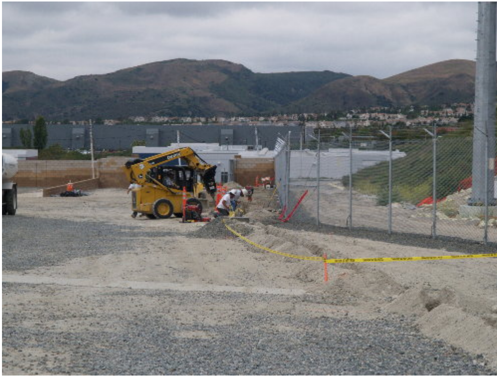
Figure 3 – KGC continued working on the trenching for the electrical needed for the light standards around the substation site.
