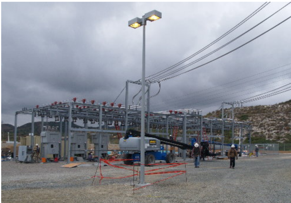
Figure 2 – NRG worked on the disconnects for the 12 kV portion of the substation.
