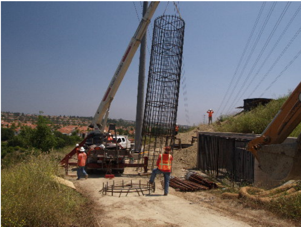
Figure 5 – The crew at H-Structure 9 removed a portion of the rebar cage to fit it into the excavation.
