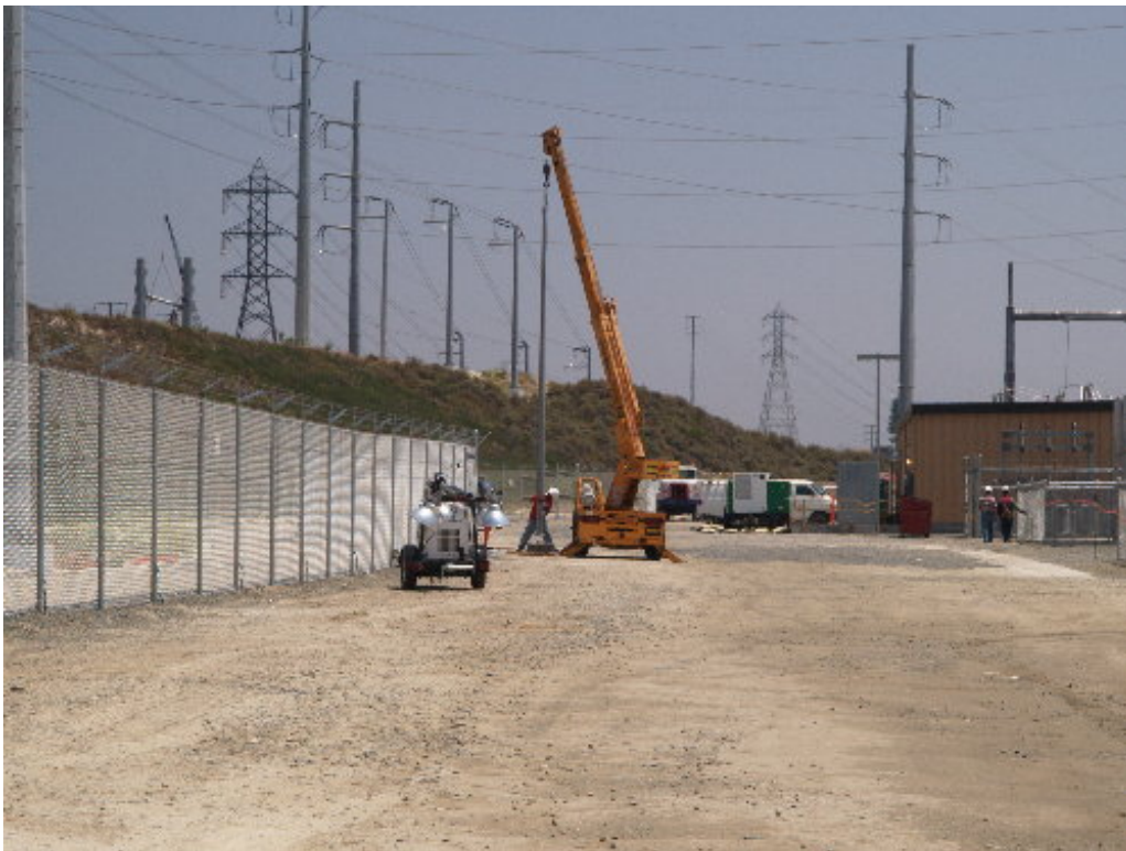
Figure 2 – A KGC crew worked with a small crane to set light poles within the substation site.
