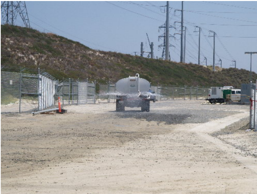
Figure 3 – A water truck was used to keep fugitive dust down within the substation site.
