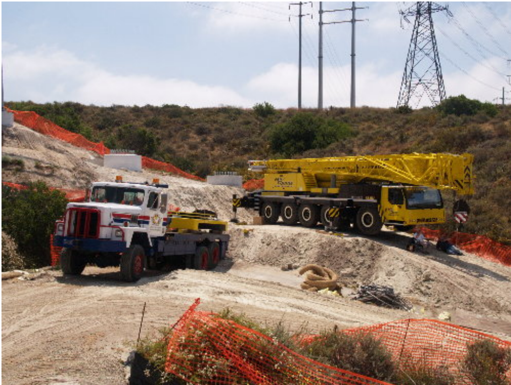
Figure 4 – The large mobile crane was staged at H-Structure 13 and will be prepared for setting the steel poles on June 15 th .
