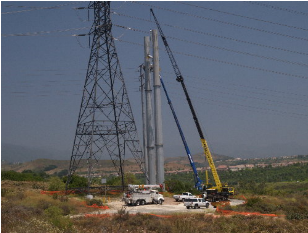
Figure 6 – Workers used a crane and a man-lift to attach the arms to H-Structure 11.
