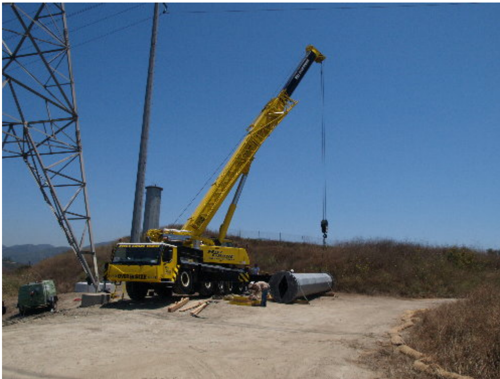
Figure 2 – Arizona crews worked with a mobile crane to set the second base for H-Structure 10.
