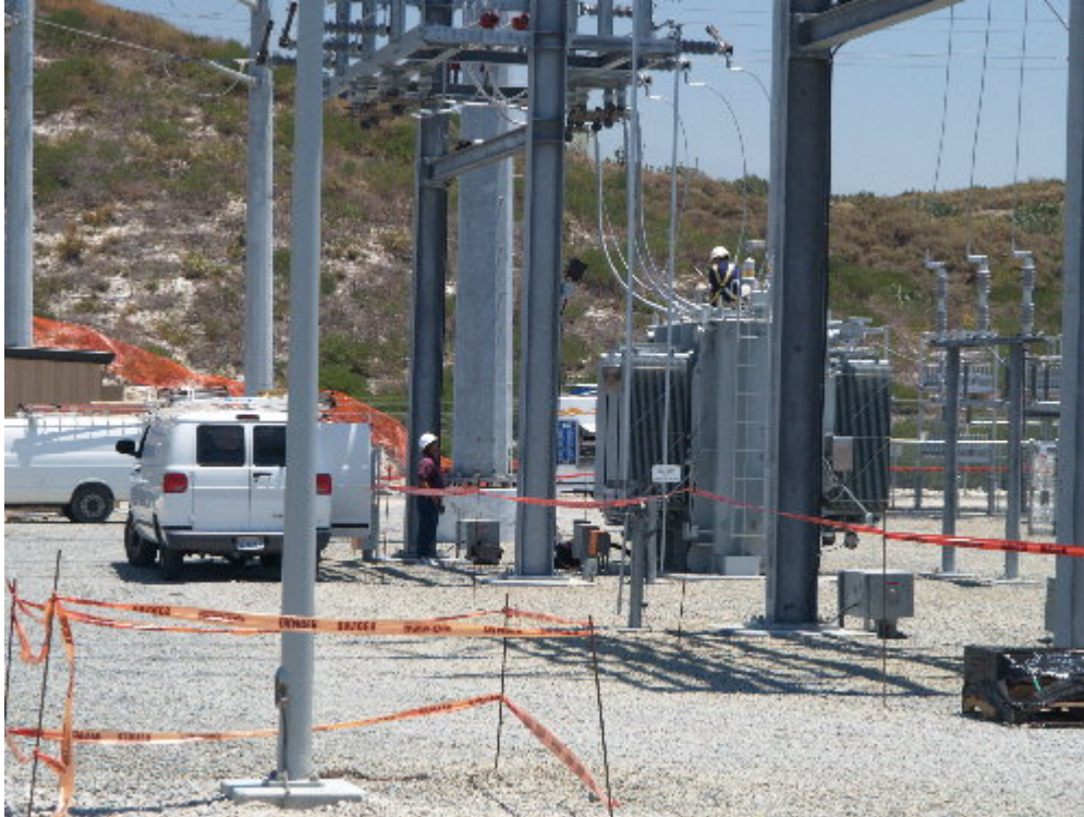
Figure 1 – NRG crews worked on the B-bank transformers during the site visit.
