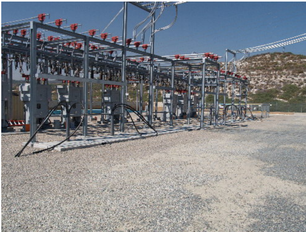
Figure 2 – The underground cables have been stubbed out at the 12 kV racks for later connection.
