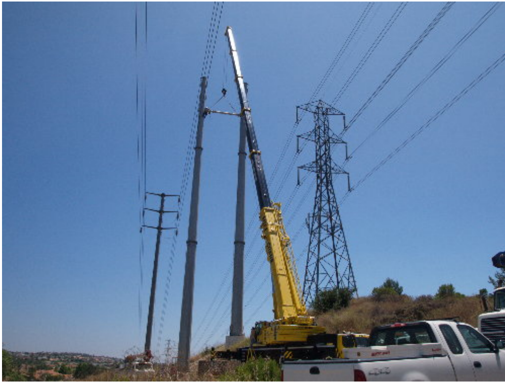
Figure 3 – Crews worked with a mobile crane at H-Structure 9 to attach the cross members.
