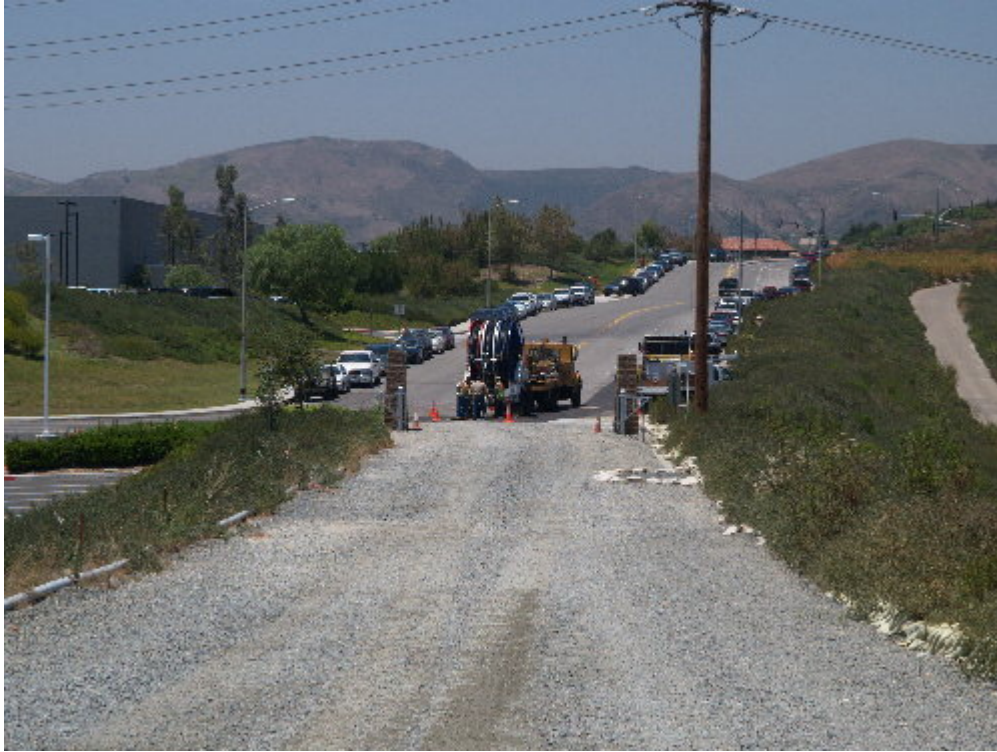
Figure 1 – A crew worked with a reel truck to pull the underground cables that will take the 12 kV power to customers.
