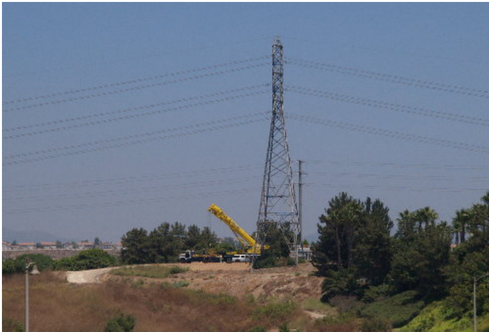
Figure 3 – The Hill Crane crew worked to prepare the mobile crane at H-Structure 8.
