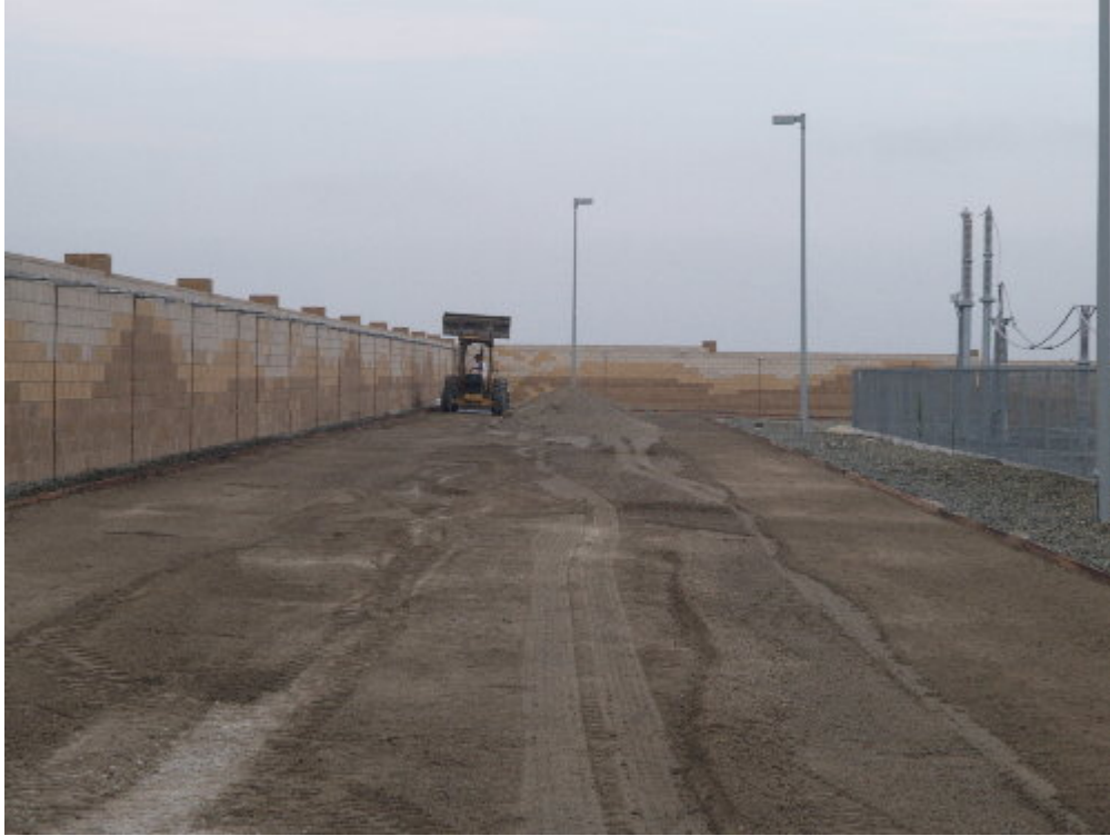
Figure 1 – The paving contractor spread base on the roadways within the substation prior to paving.
