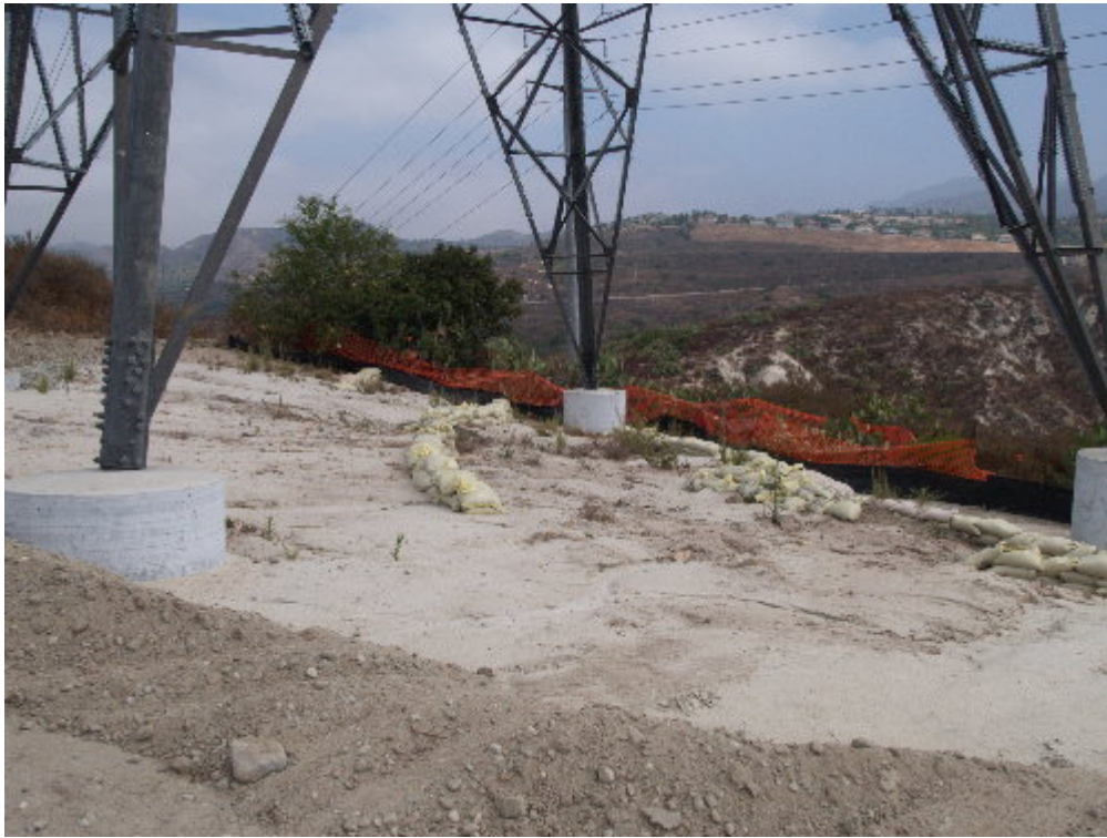
Figure 3 – The non-native plants were removed at the 220 kV structure above the substation site.
