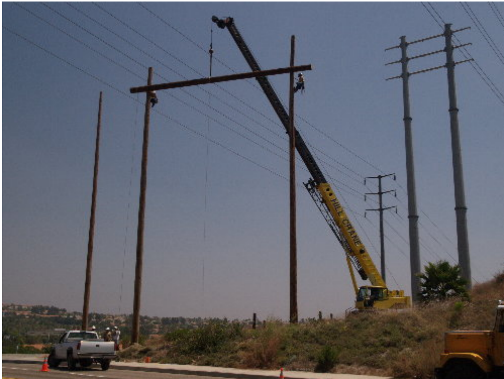
Figure 4 – An SCE transmission line crew worked to set the guard structure on Aliso Parkway.
