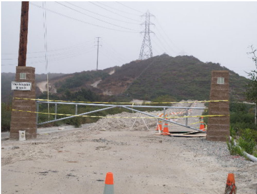
Figure 2 – No progress has been observed on the water line to the substation.
