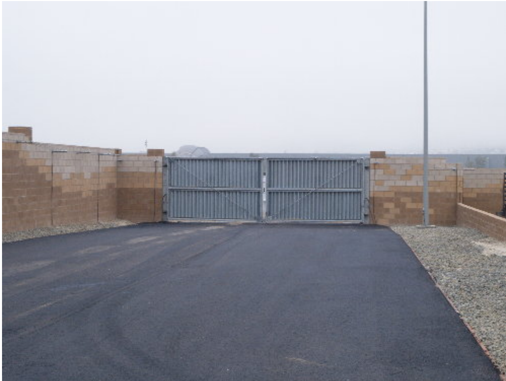
Figure 1 – The paving crew completed the asphalt and the gate at the northwest corner of the substation site has been installed.
