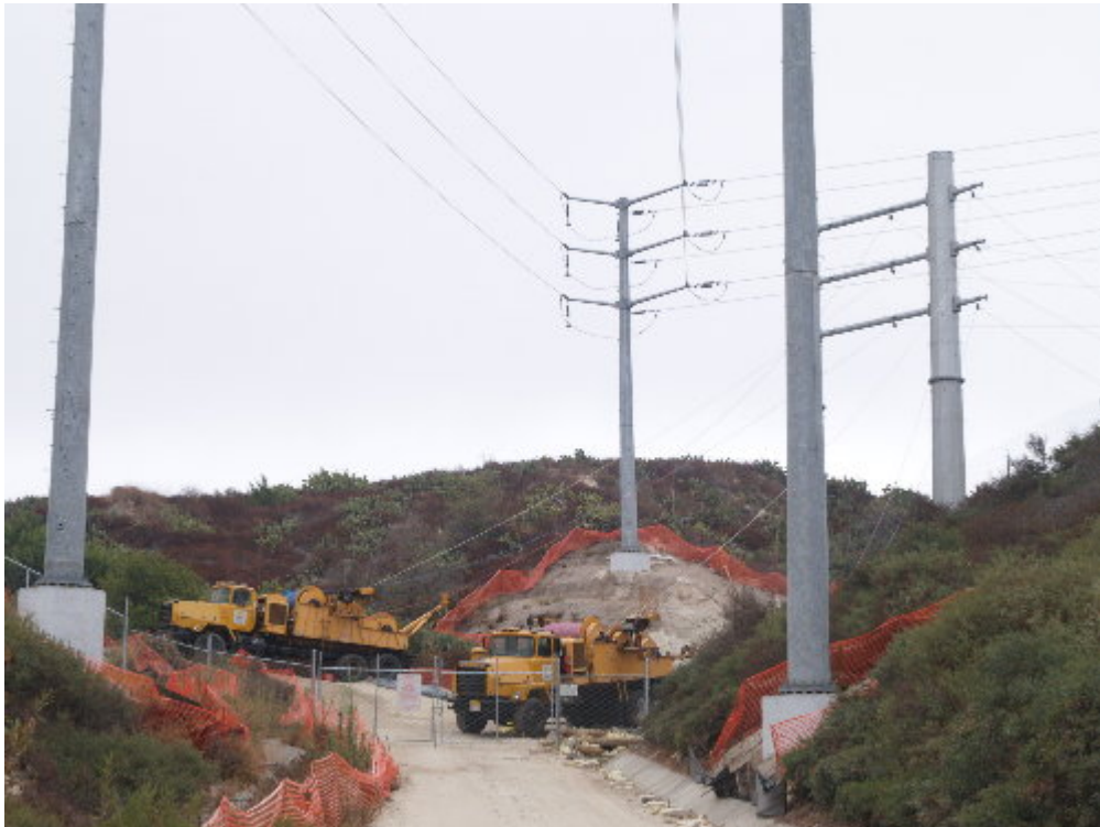
Figure 3 – Reel trucks were stationed at H-Structure 13 to pull conductor between the 241 toll road and the substation site.
