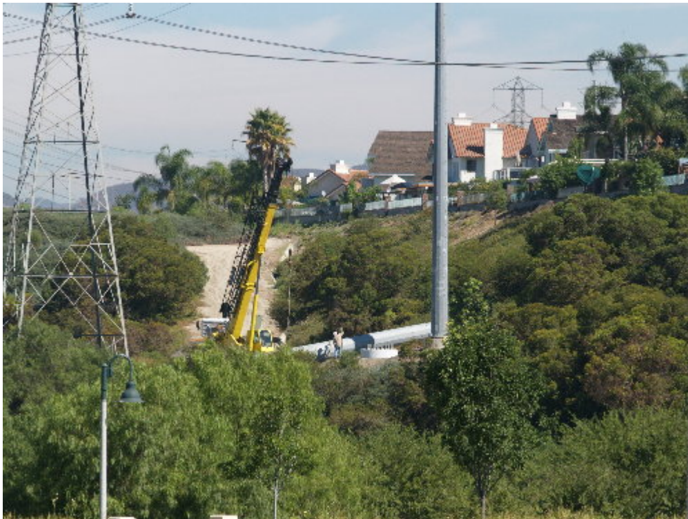
Figure 2 – The crane was set up at H-Structure 4 and the crew prepared to raise the steel pole sections.
