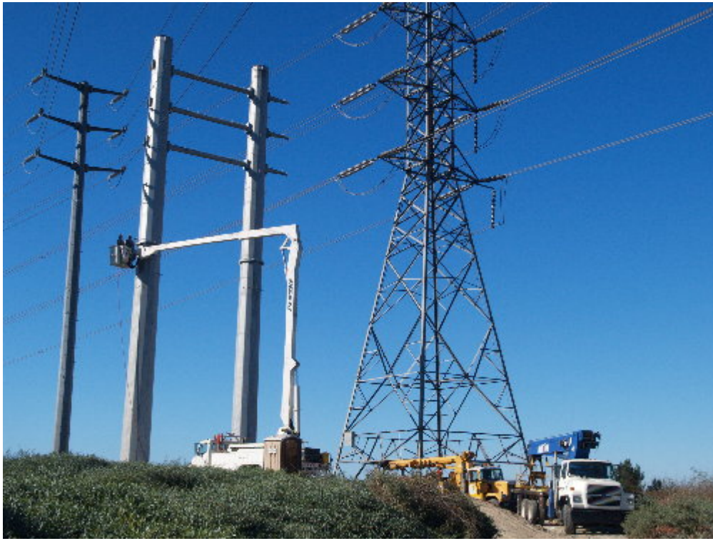
Figure 3 – The crew at H-Structure 5 worked to tighten the bolts on the arms.
