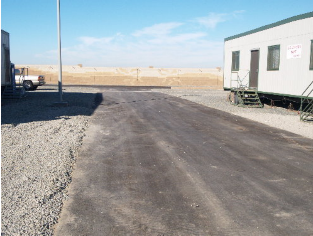
Figure 1 – The gravel has been laid on the apron of the new roads within the substation site.
