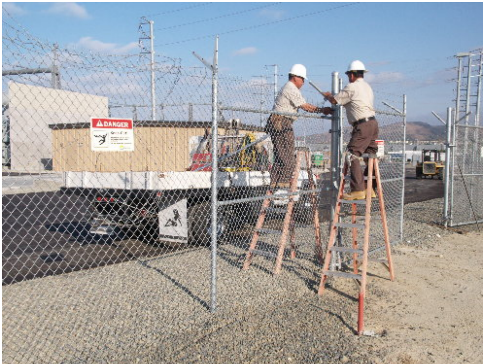
Figure 2 – The fencing subcontractor repaired damage to the eastern fence during the site visit.
