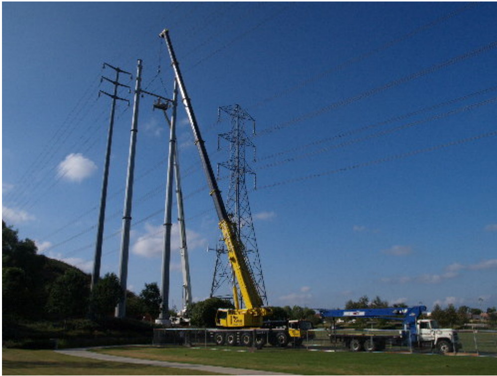
Figure 3 – The SCE transmission line crew worked to attach the cross-members to the H-Structure in Olympiad Park.
