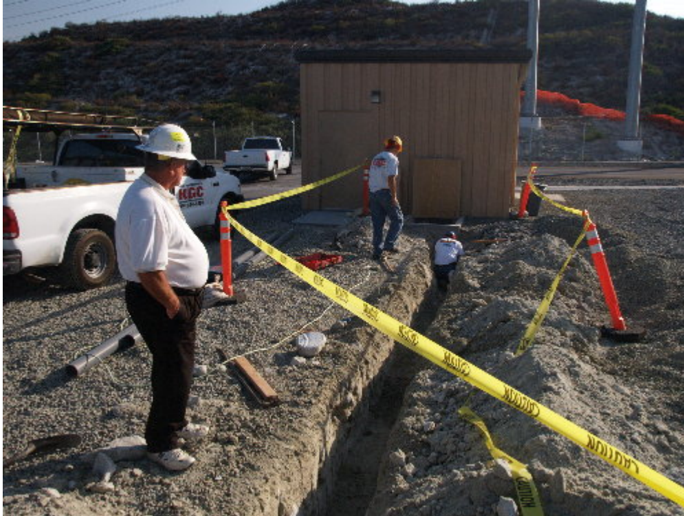
Figure 1 – KGC trenched west from MEER #2 to install fiber optic cable that will monitor the temperature of the underground conduit.
