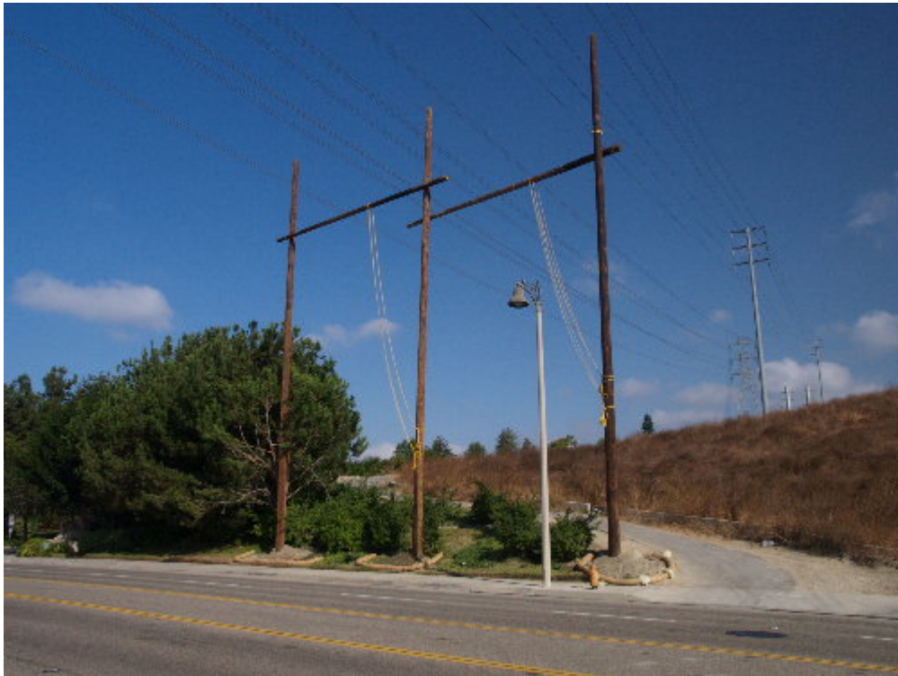
Figure 4 – BMPs have been placed at the base of the guard structures.
