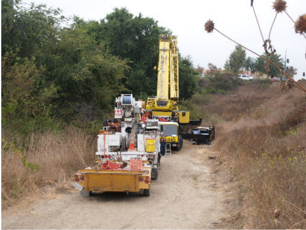
Figure 1 – A crew worked to prepare the larger crane for mobilization from the site.
