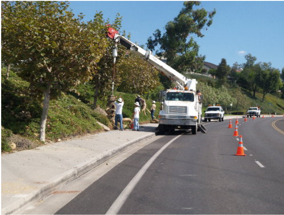
Figure 2 – The transmission line crew used a truck mounted auger and hand tools to excavate for the guard structures.
