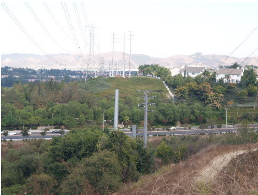
Figure 1 – One pole section and the arms remain to be installed a Structure 1.
