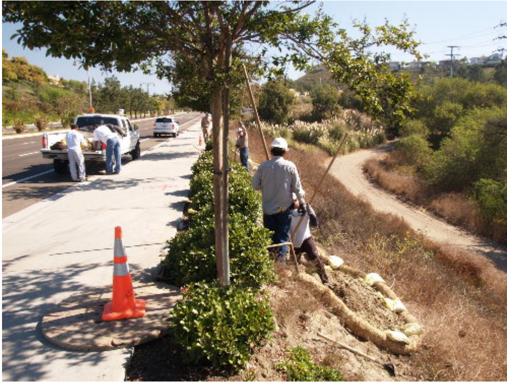
Figure 1 – The transmission line crew used a truck mounted auger and hand tools to excavate for the guard structures.
