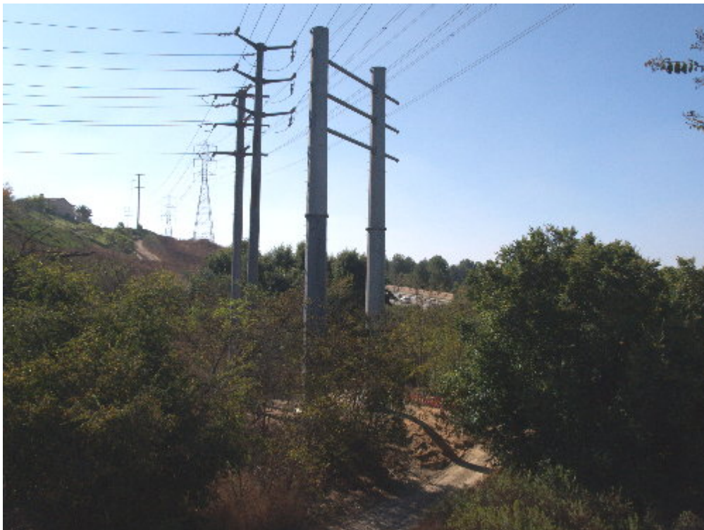
Figure 2 – The remainder of H-Structure 1 has been raised. The remaining arms will be attached once the other line has been removed.
