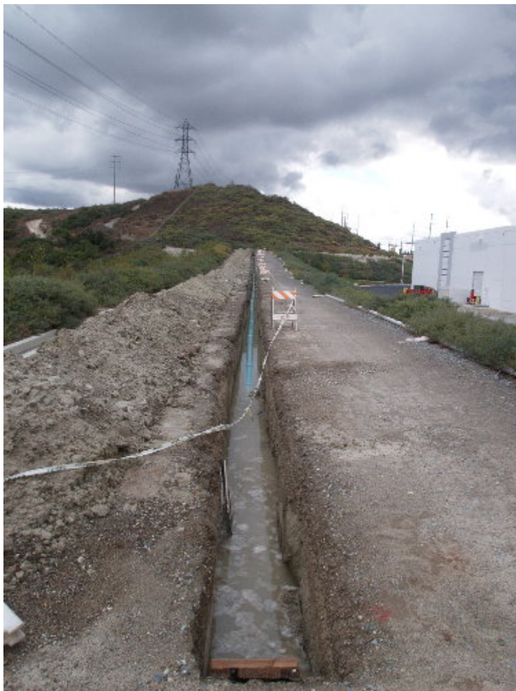
Figure 1 – The open trench on the main entrance to the Viejo Substation has partially filled with water.
