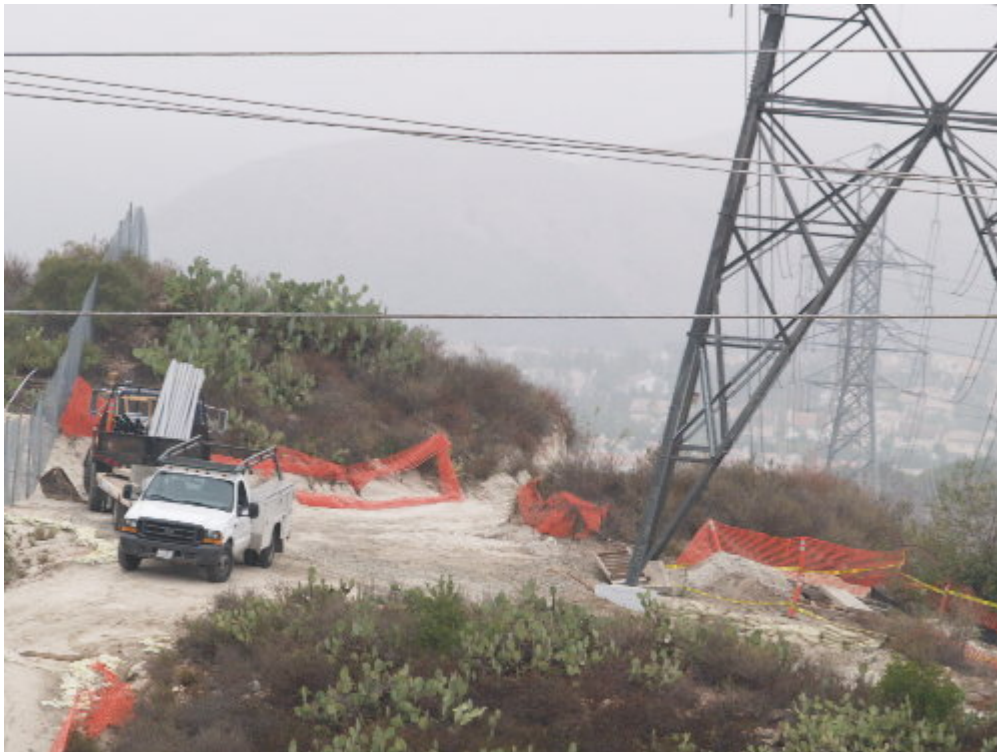
Figure 2 – A crew unrelated to the Viejo System Project installed communication conduit in the SCE right-of-way above the Viejo Substation.
