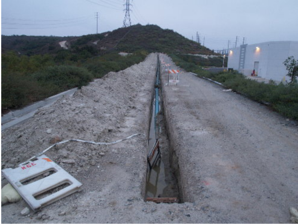
Figure 1 – The open trench on the main entrance to the Viejo Substation has partially drained, but water remains. Some of the pipe is now covered with silt.
