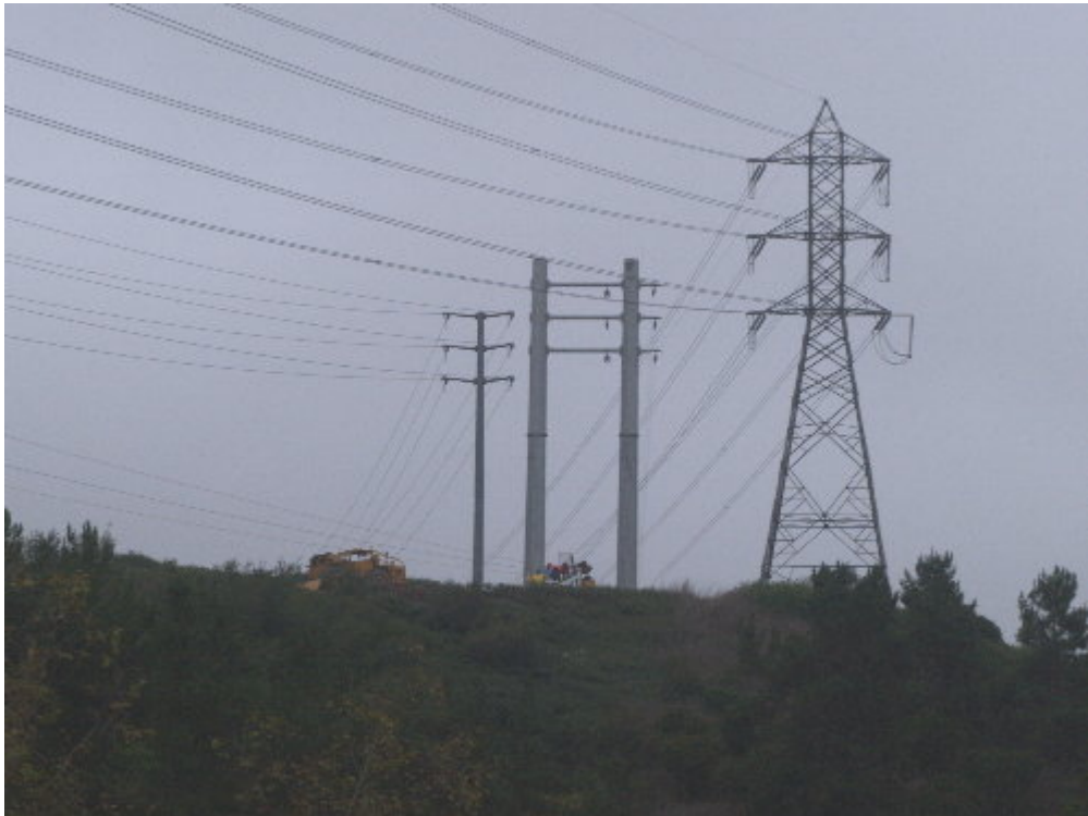
Figure 4 – SCE crews worked to pull conductor between Structures 7 and 5 during the site visit.
