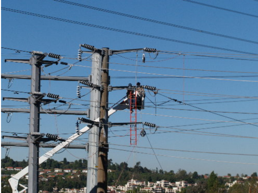
Figure 1 – A crew set up adjacent to H-Structure 1 with a boom truck to support the crew wrecking out the old conductor on the 66 kV steel pole.
