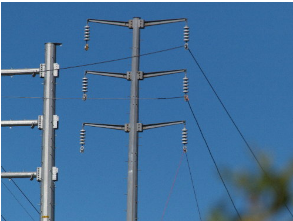
Figure 2 – The center conductor on the old 66 kV steel poles has been spliced with rope for wrecking out. The bottom conductor has already been removed.
