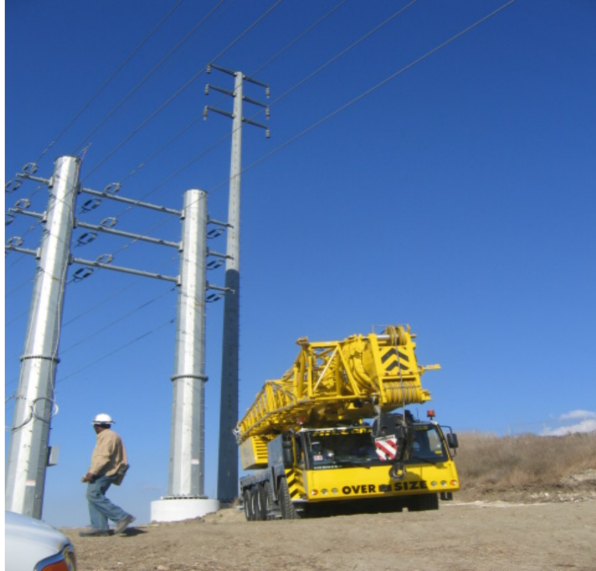
Figure 1 – Crew prepares to dismantle and remove an old 66 kV steel pole along the right-of-way, December , 2005.
