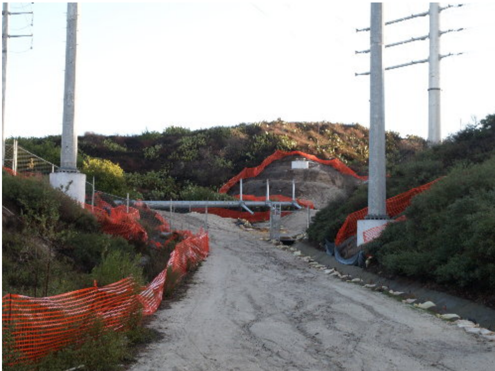
Figure 2 – The temporary steel pole adjacent to H-Structure 13 was lowered and will be removed.
