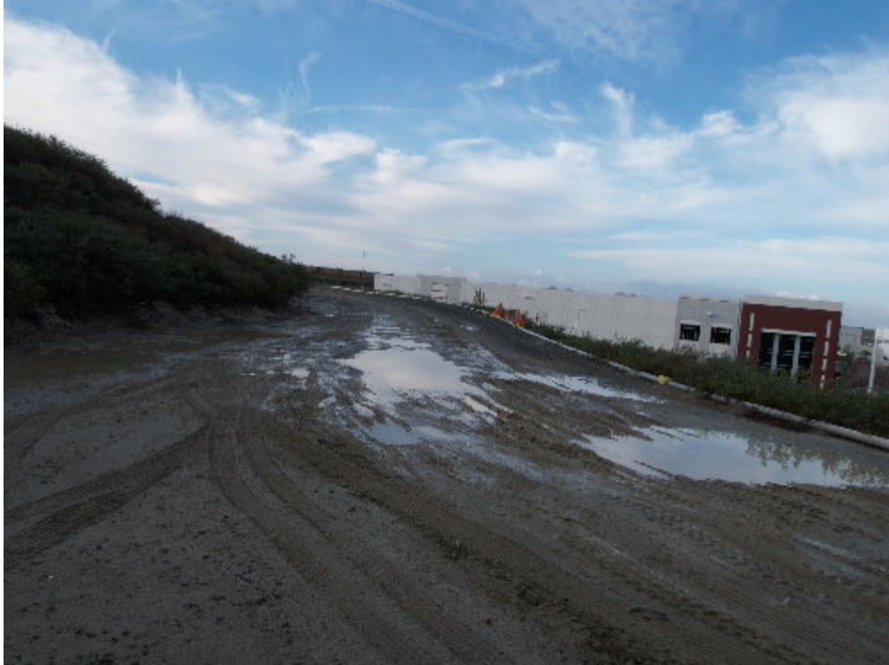
Figure 1 – The main road to the substation has been backfilled and was muddy during the site visit.
