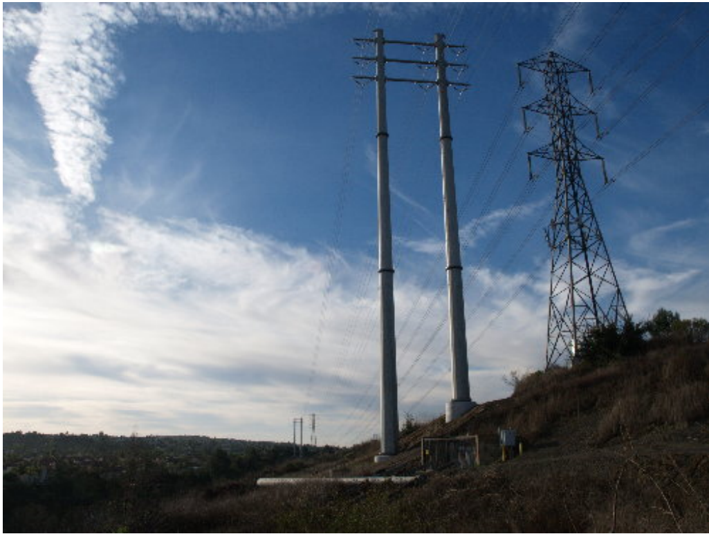
Figure 3 – The old steel poles have been lowered, but many are still on the right-of-way. These poles will be removed once the access roads dry out from the recent rains.
