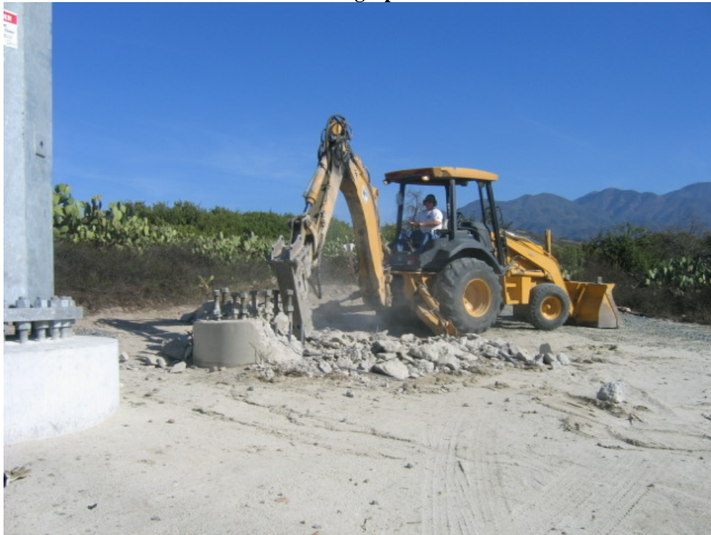
Figure 1 – Arizona Pipeline crew dismantling a tower footing above the Viejo Substation during the site visit.
