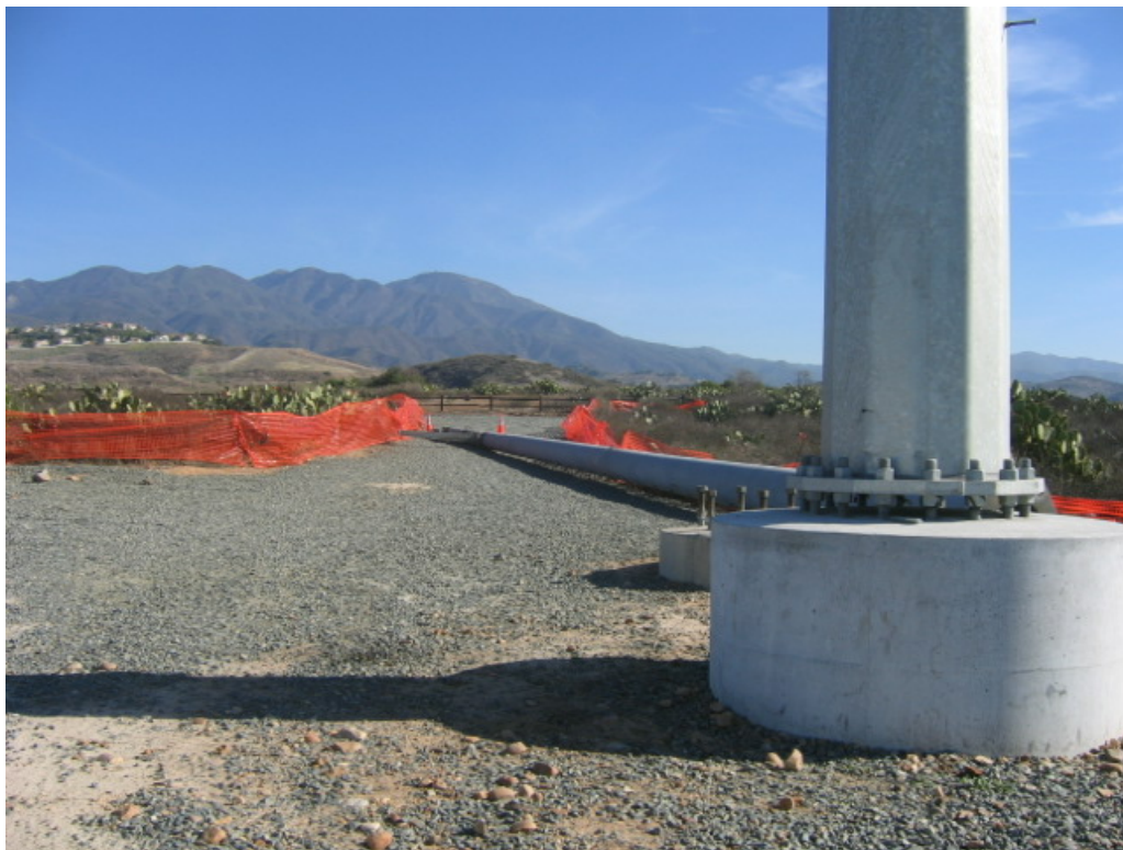
Figure 2 – The old steel pole will be cut up and removed from the project area.
