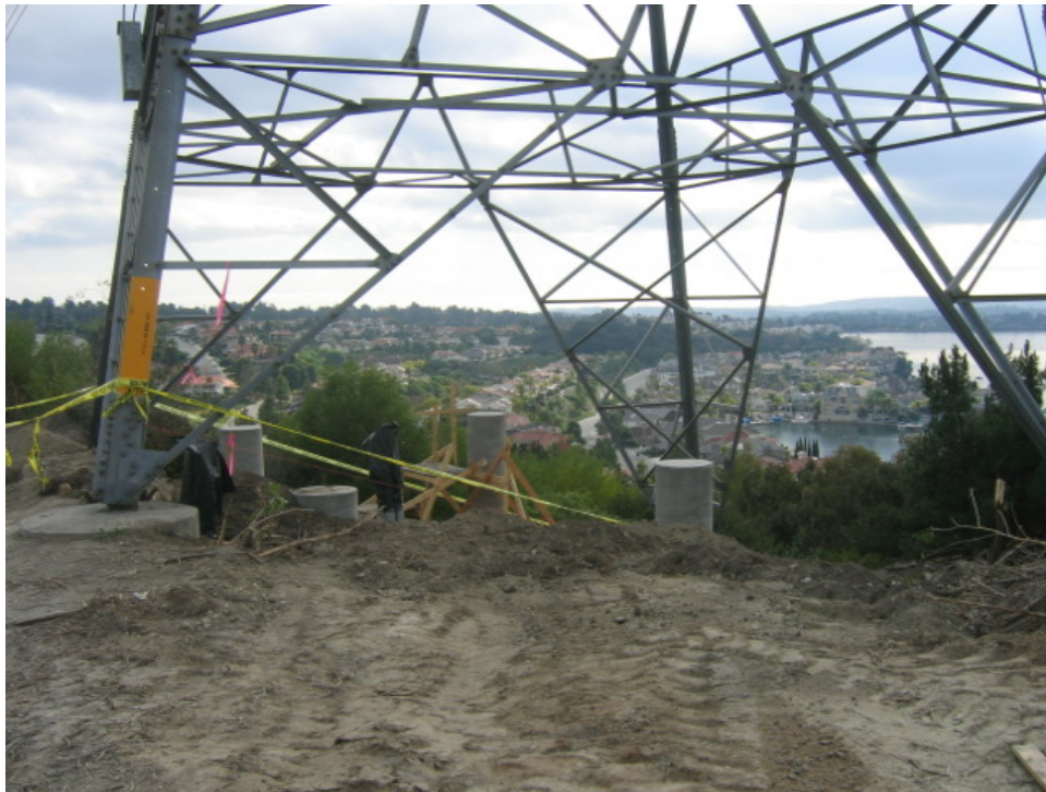
Figure 2 – Fiber optic vault structure construction at a lattice tower within the SCE right-of-way.
