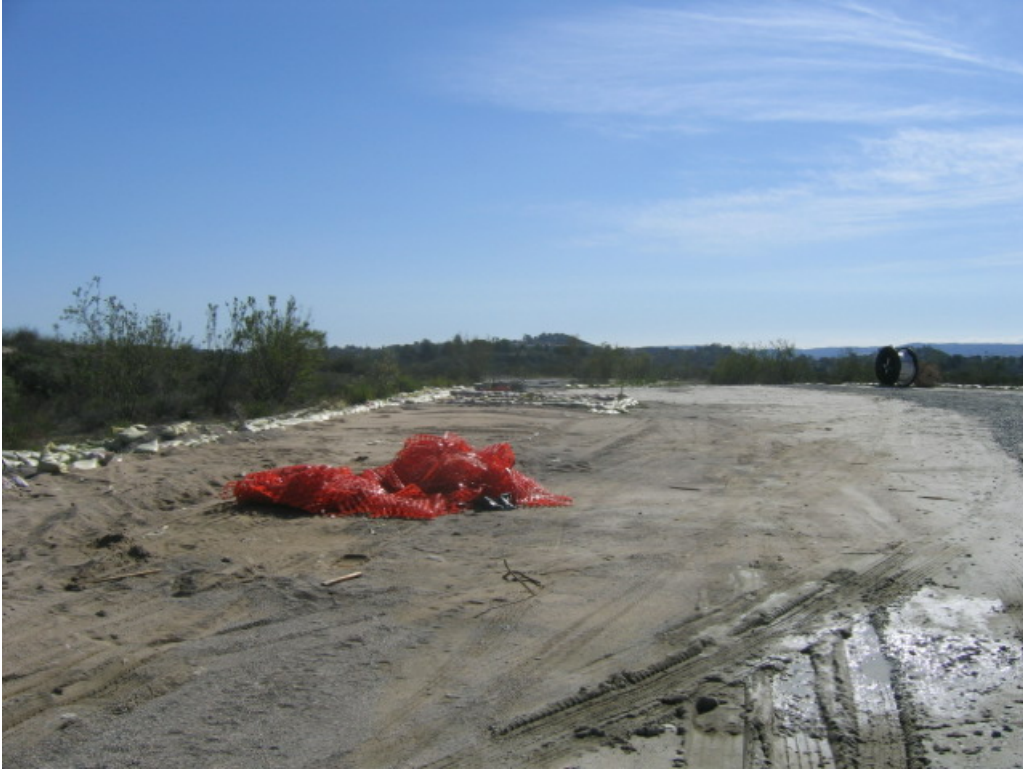
Figure 1 – Area behind the Viejo Substation used for staging materials. Most project materials have been removed.
