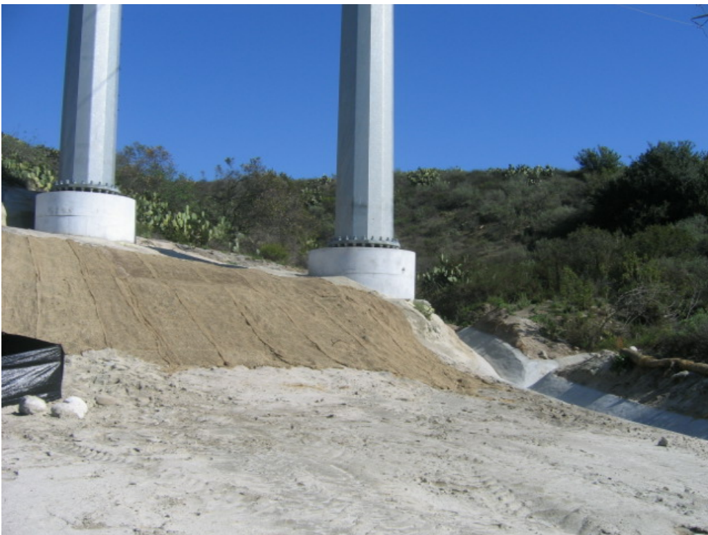
Figure 2 – Restoration of a tower pad under H structure near Viejo Substation. Note the new v-ditches and erosion netting.
