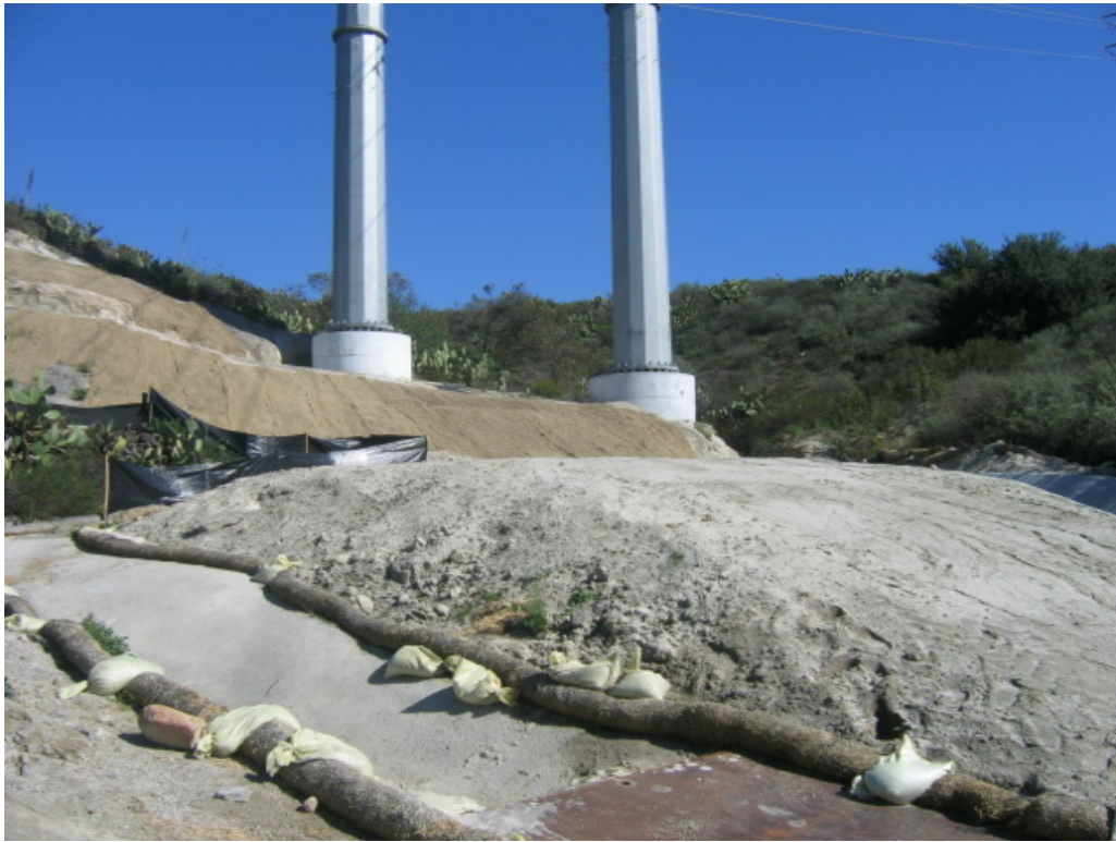
Figure 3 – Restored area near Viejo Substation. SCE crews routinely check the right-of-way for erosion and BMP repair.
