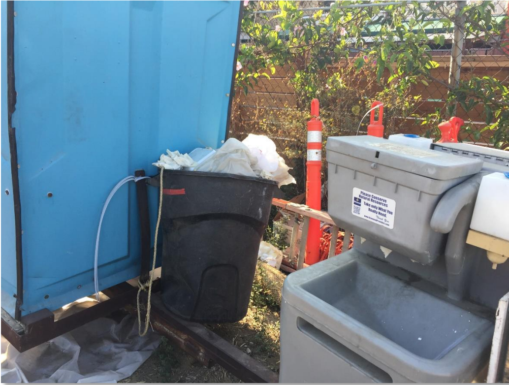
Photo 20. Uncovered and overflowing trash container stored for the 12 kV underground crews along India Street
