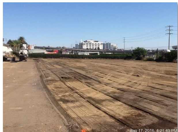
Photo 2. Removal of the asphalt from the substation site, previously used as an airport parking lot
