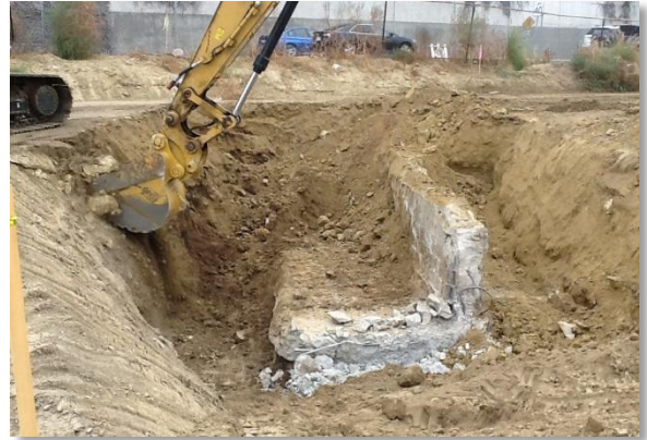
Photo 3. After the unmarked foundation was evaluated, the crews continued to remove the feature
