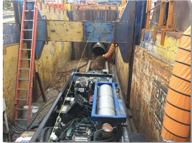
Photo 12. Equipment set of for the jack and bore under the railroad right of way
