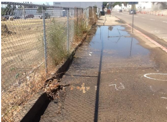
Photo 7. Flooding after the accidental hydrant disconnection along Kettner Boulevard
