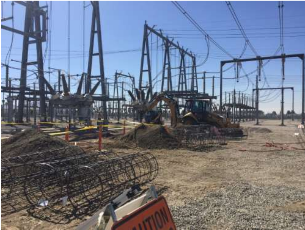
Figure 1 – Construction crews removed existing foundations and drilled holes for new foundations for the replacement switch racks.
