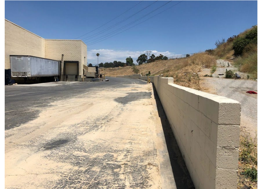
Photo 6. Sediment deposits from water line break at 2N30 prior to clean-up (July 11, 2019)
