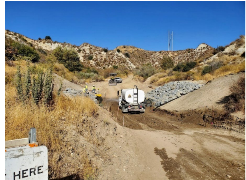
Photo 8. Grading activities at wet crossing on access road to Construction Area 4X04, Segment 4 (October 12, 2020)
