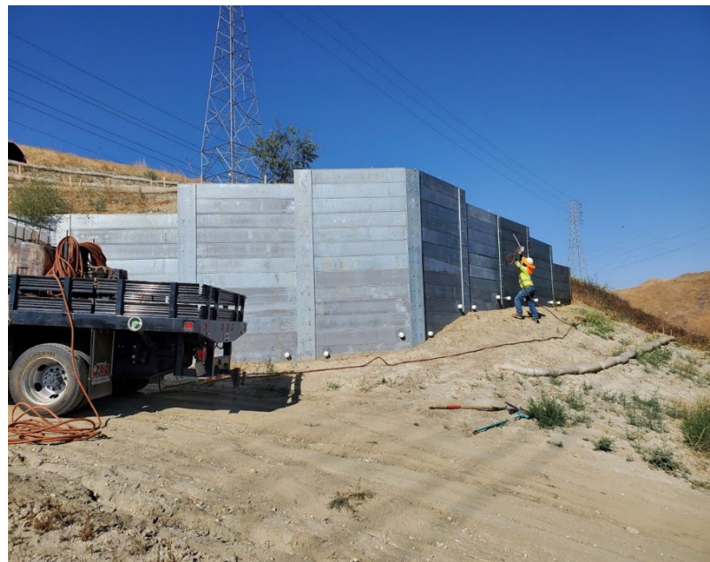
Photo 12. Natina application to soldier pile wall at Construction Area 2N11, Segment 2 (June 21, 2021)
