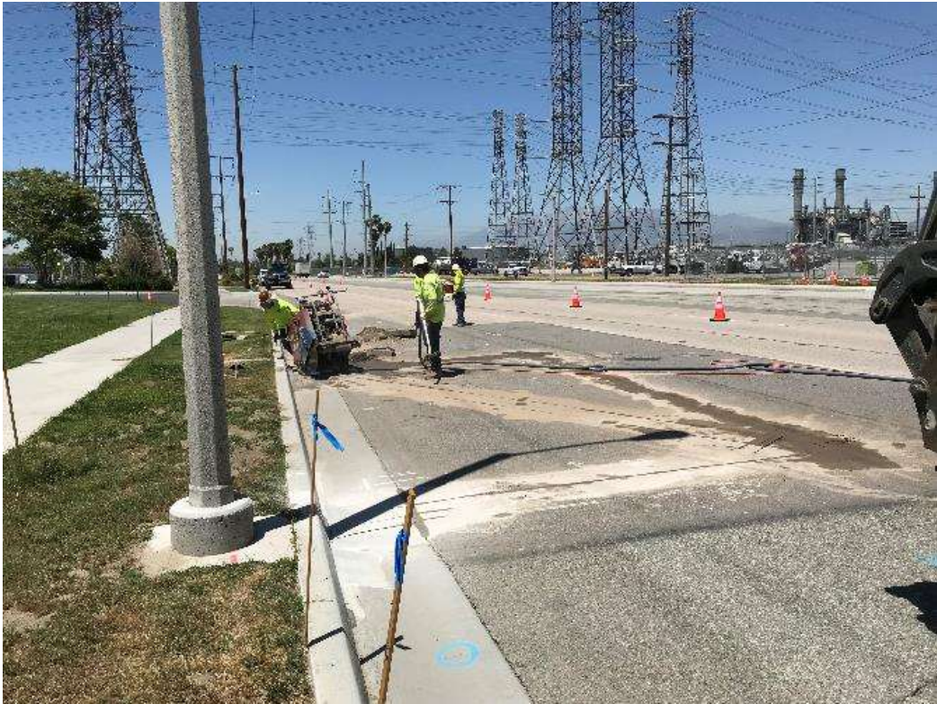
Photo 4 – Asphalt cutting prior to vault excavation along San Bernardino Avenue for Timoteo Relocation (May 7, 2018).
