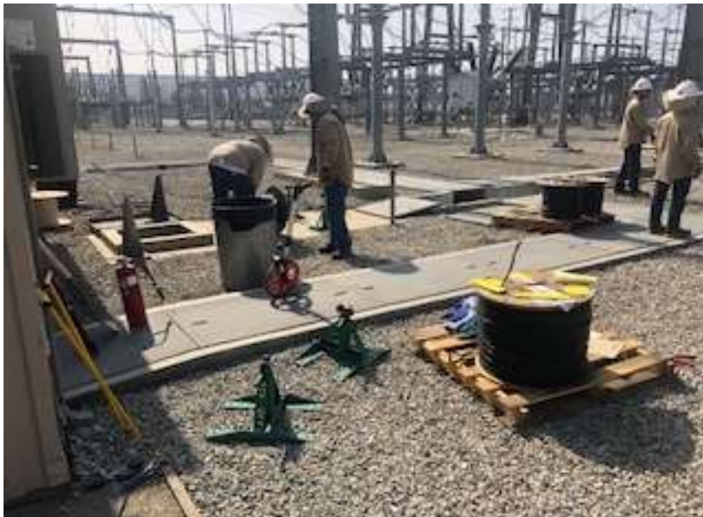
Photo 2 Installing cable at the San Bernardino Substation (photo courtesy of SCE FRED) (June 8, 2018).
