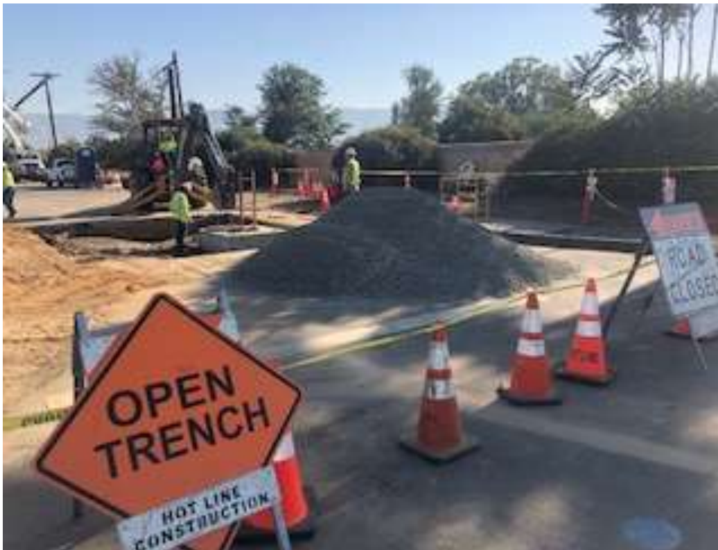
Photo 3 – Vault installation occurring along Iowa Street for the Tennessee Relocation (photo courtesy of SCE FRED) (May 30, 2018).
