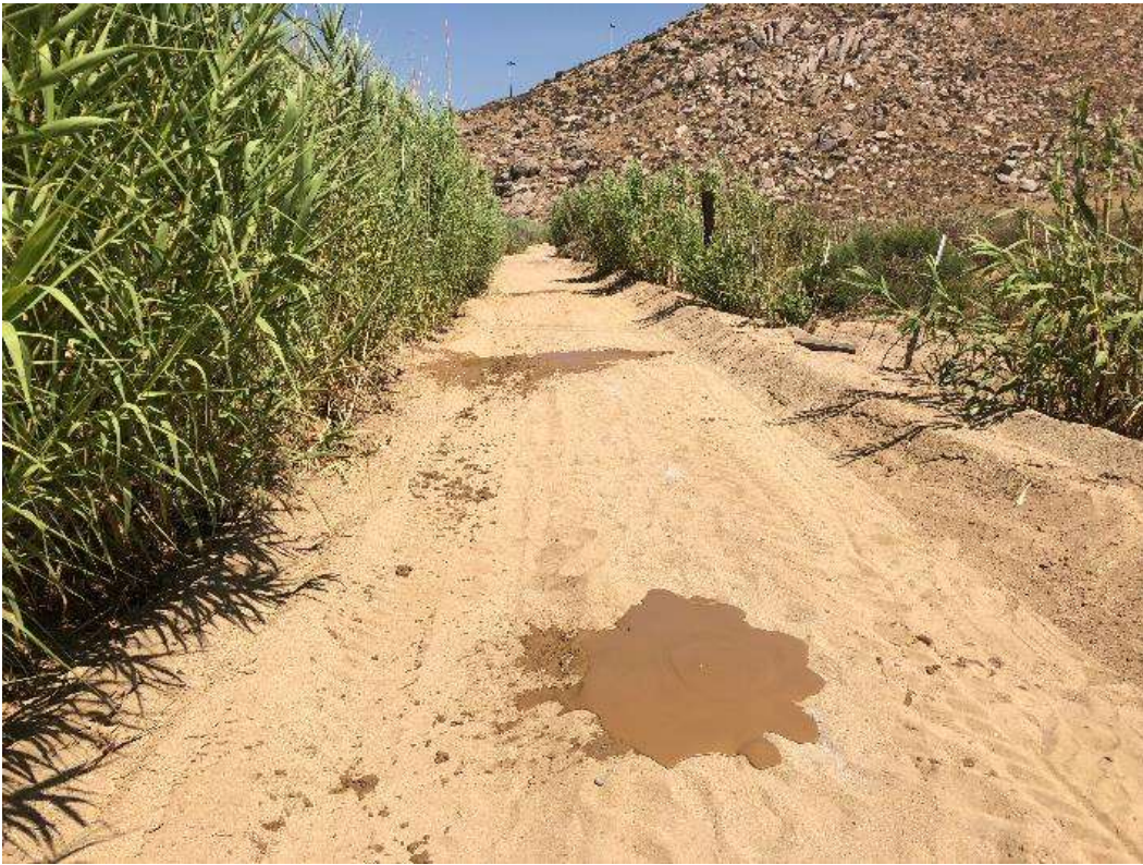
Photo 7 – Three additional frac-outs identified along Smith Creek during HDD operations (August 14, 2018).
