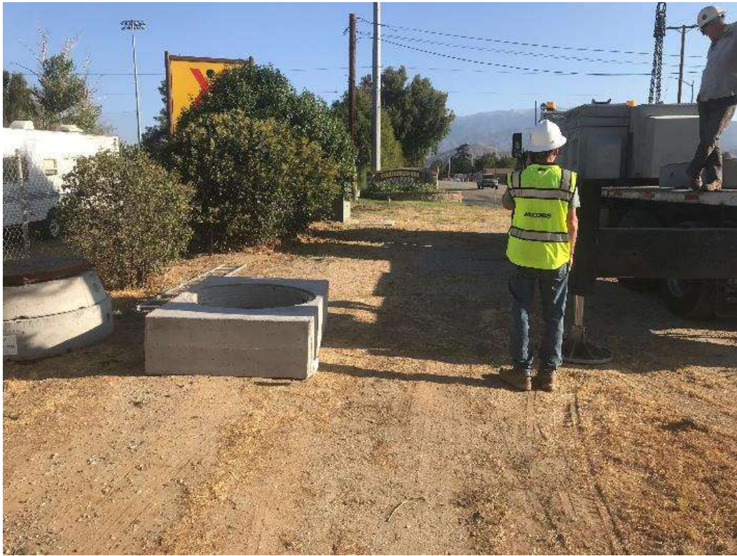
Photo 5 – HDD crew unloading manhole cover in unapproved work area (August 14, 2018).
