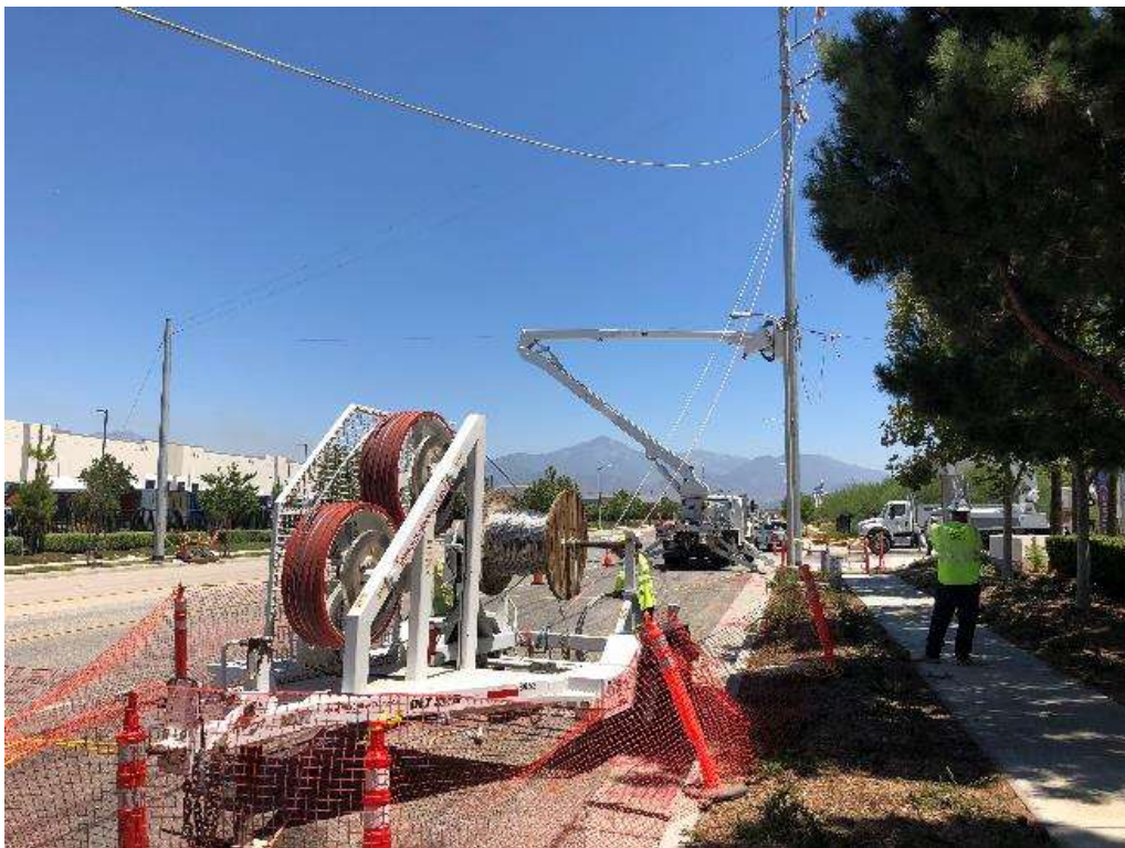
Photo 2 – Installing overhead conductor wire along Lugonia Avenue for the Timoteo Relocation (August 6, 2018).
