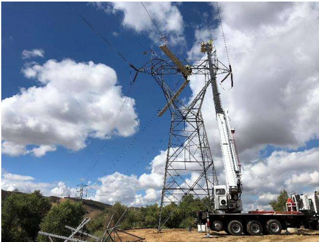
Photo 5 – Abercrombie crew wrecking out wire from existing tower at Site 4N62, Segment 4 (October 4, 2018).
