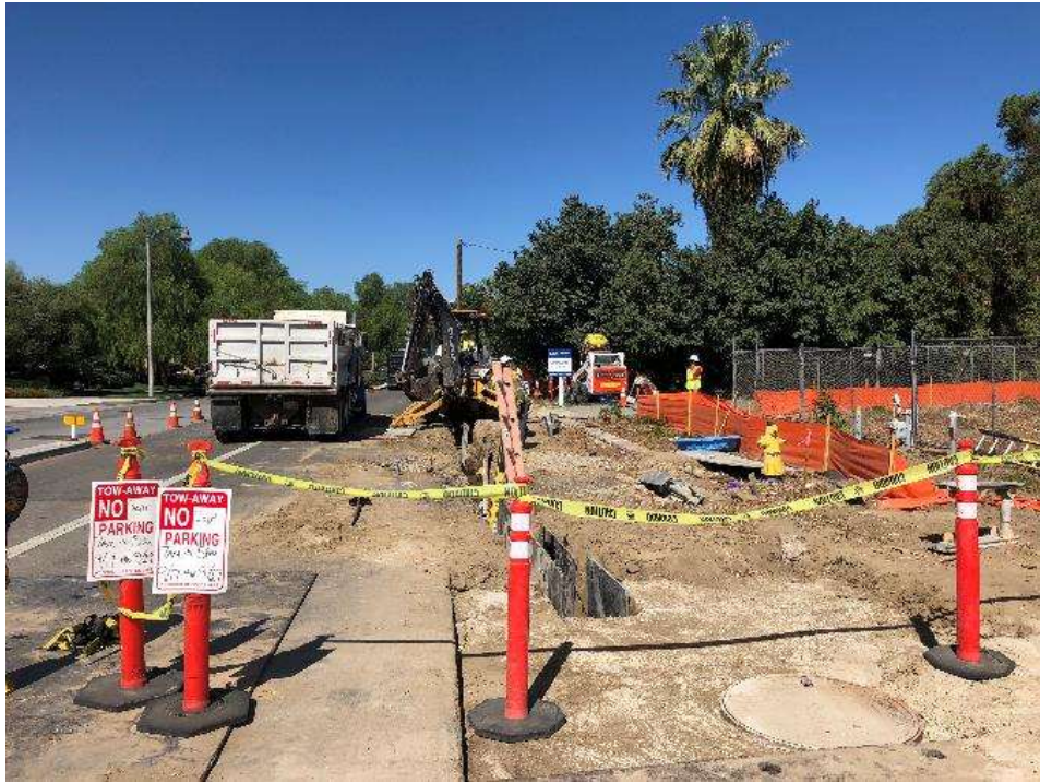
Photo 1 – Trenching and conduit installation along Mission Avenue for the Dental/Intern Circuits (October 1, 2018).
