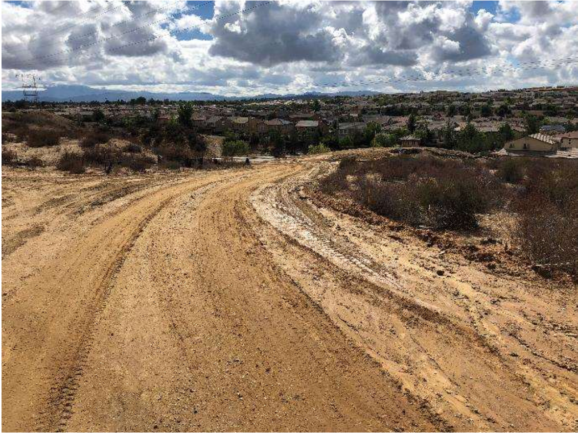
Photo 7 – Minor erosional rills along access road near Site 4X51, Segment 4. CPUC EM confirmed that additional sandbags had since been installed (October 4, 2018).
