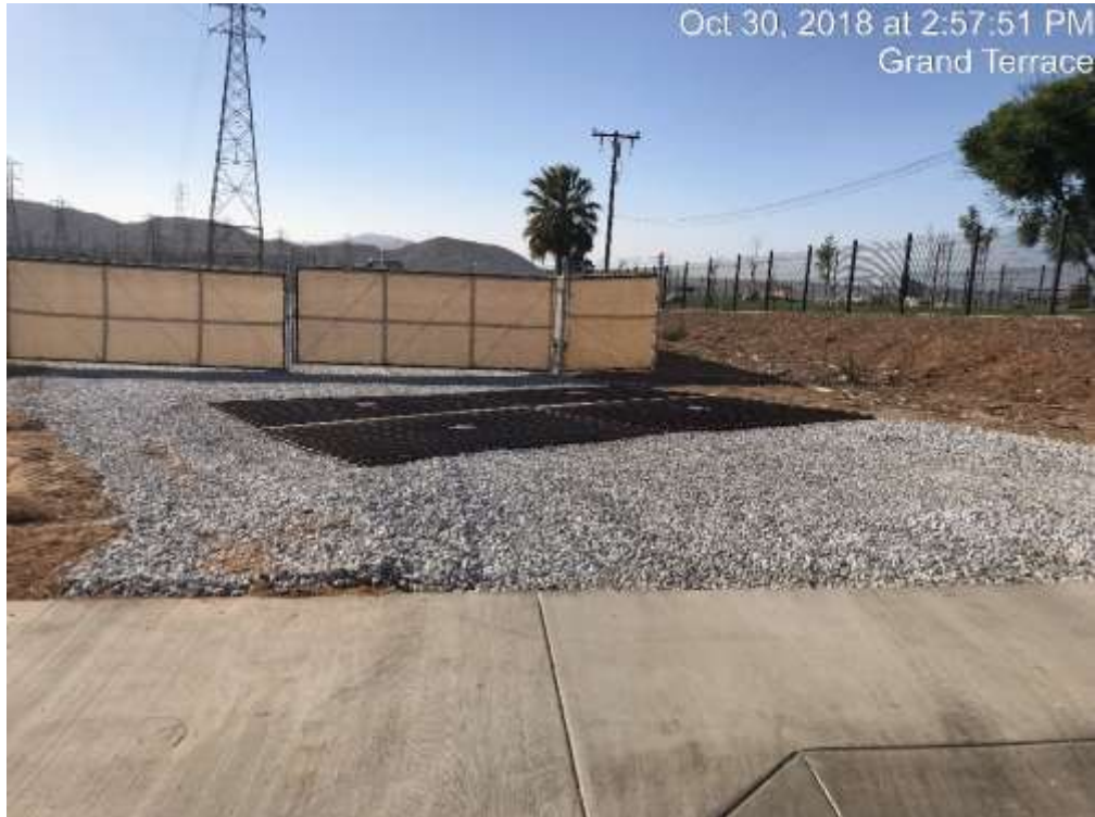
Photo 1 – Grand Terrace Yard had a stabilized entrance installed to prevent track-out and dust. (October 30, 2018).
