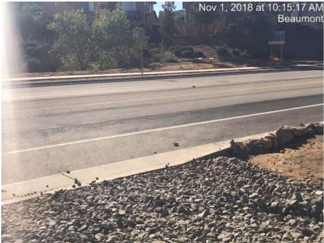
Photo 5 – Track out of rock onto Palmer Ave was reported by the CPUC EM (November 1, 2018).
