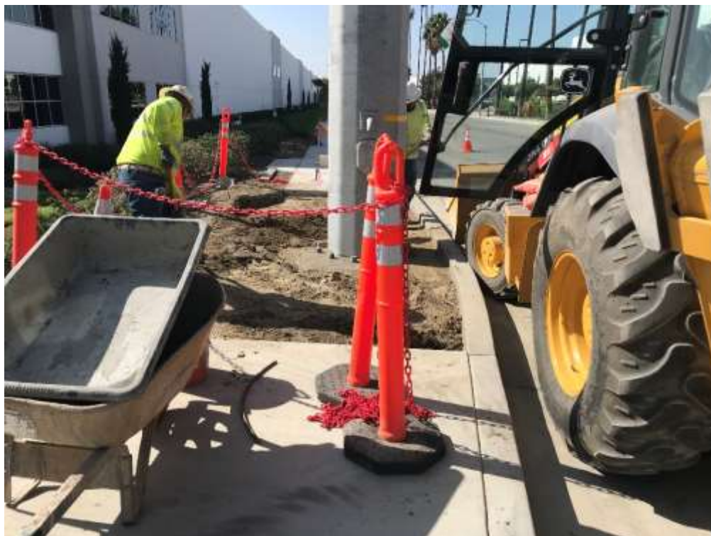
Photo 2 – Sidewalk restoration following pole placement along Nevada Street for the subtransmission work performed by Hotline Construction (October 30, 2018).
