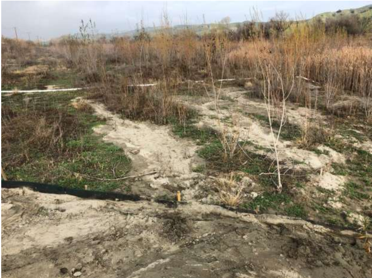
Photo 4 – Offsite sedimentation after recent rain events at Tower 4N63, Segment 4. Sediment from the graded tower side overlook BMPs and discharged sediment into the adjacent jurisdictional drainage. USACE, CDFW, and SWRCB were notified by SCE. Photo courtesy of SCE.
