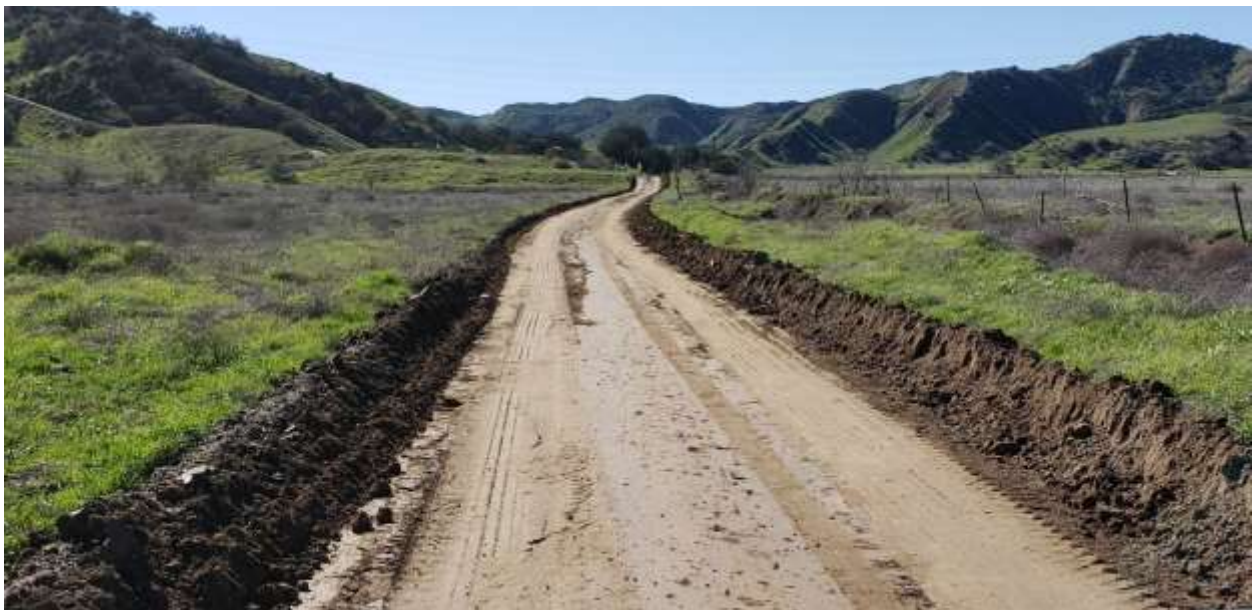
Photo 2 – Crews conducted access road grading in areas of Segment 3 to allow of equipment access to tower sites during and following rain events.
