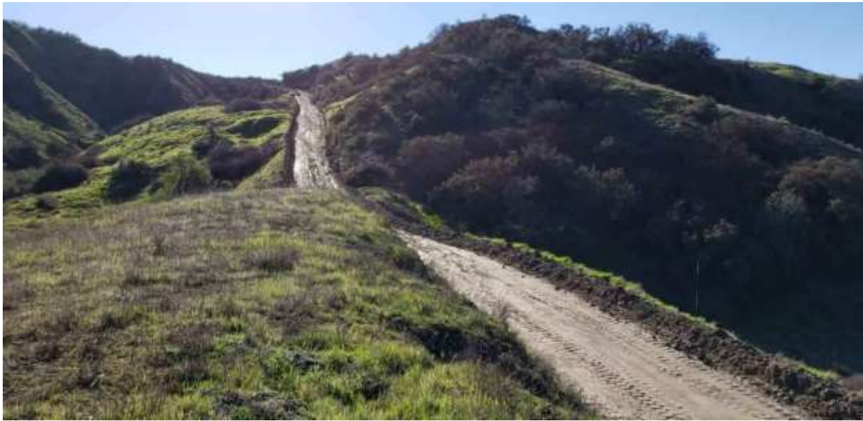
Photo 3 – Access road grading to facilitate project equipment accessing work sites in Segment 3.
