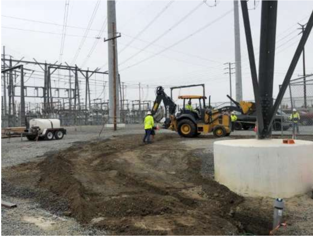
Photo 1 – Conduit installation activities at Construction Area 1X26, Segment 1 (June 19, 2020) (Photo courtesy of SCE).
