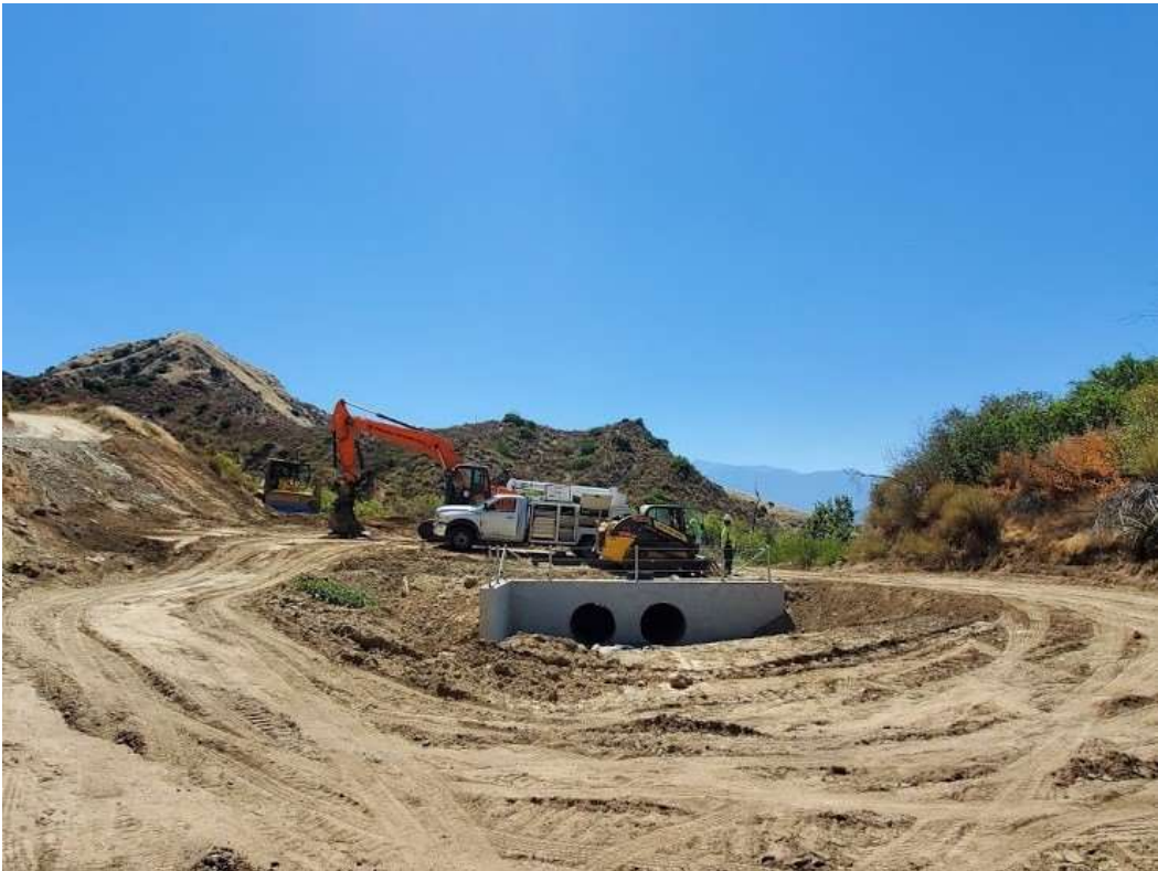
Photo 4 – Construction activities at drainage crossing on access road to Construction Area 4X04, Segment 4 (July 21, 2020).
