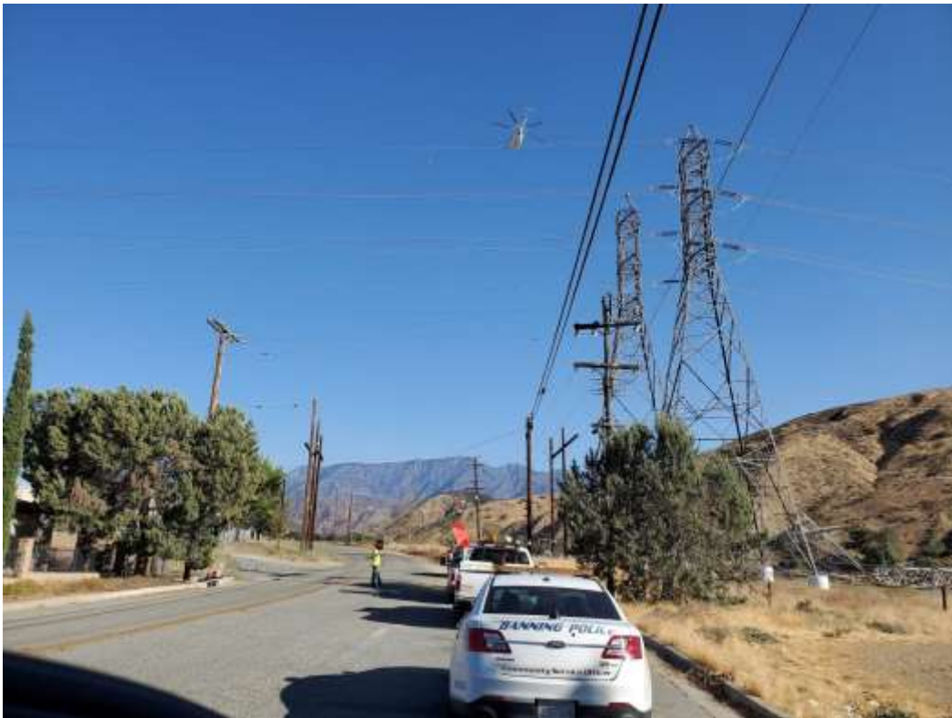
Photo 5 – Wire stringing activities with traffic control at Construction Area 4X01, Segment 4 (September 30, 2020).
