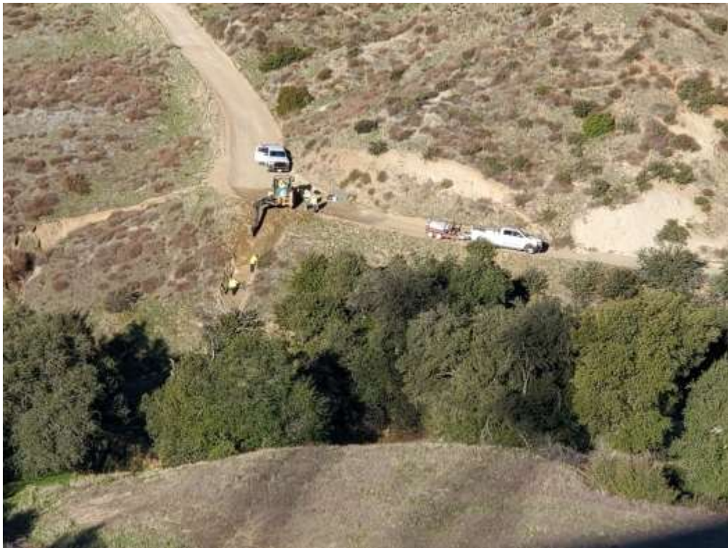
Photo 5 – MAC drain vegetation clearing and installation at Construction Area 4X12, Segment 4 (February 24, 2021).
