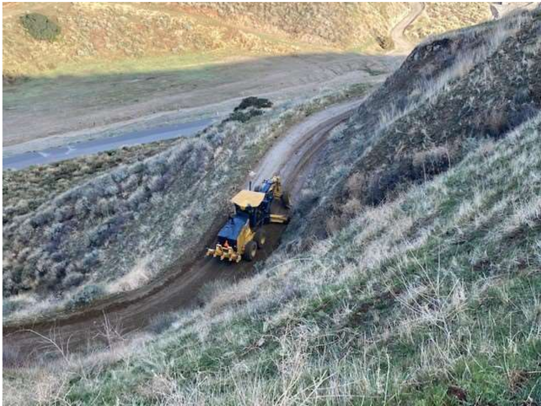
Photo 4 – Access road maintenance on Smiley Road, Segment 3 (Photo courtesy of SCE) (March 12, 2021).
