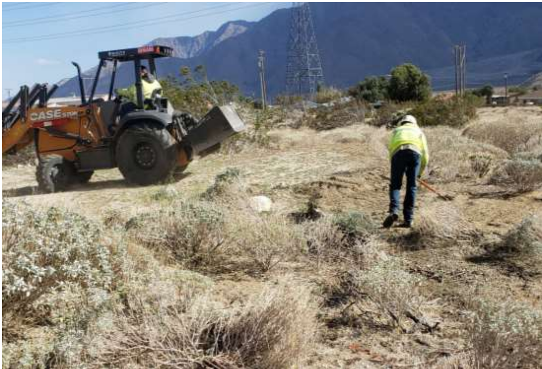
Photo 6 – Site scarification at Construction Area 6N40, Segment 6 (Photo courtesy of SCE) (March 9, 2021).
