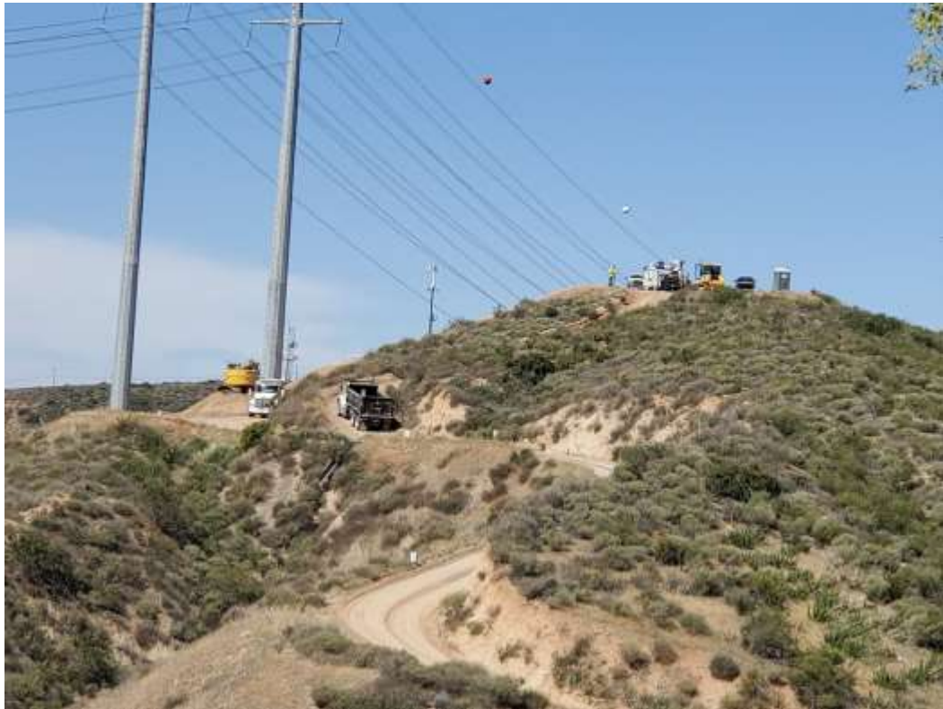
Photo 4 – Tower pad recontouring and soil export at Construction Area 4X03, Segment 4 (May 5, 2021).
