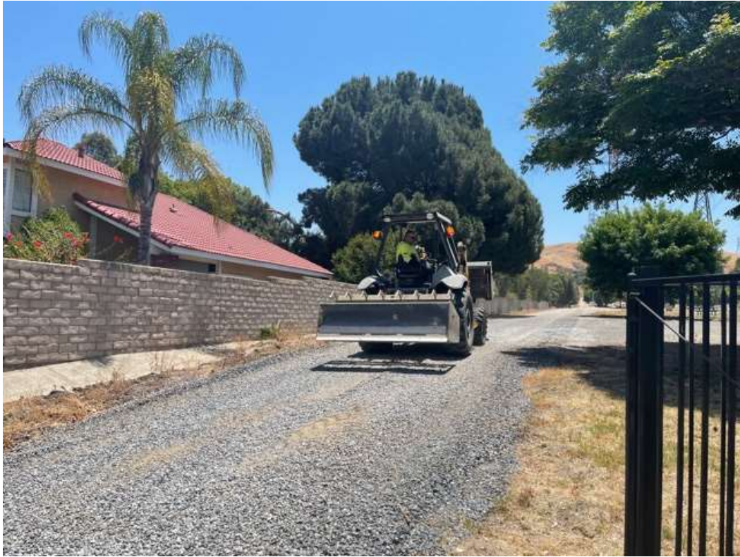
Photo 1 – Construction entrance removal at Construction Area 1X05, Segment 1 (June 3, 2021) (Photo courtesy of SCE).
