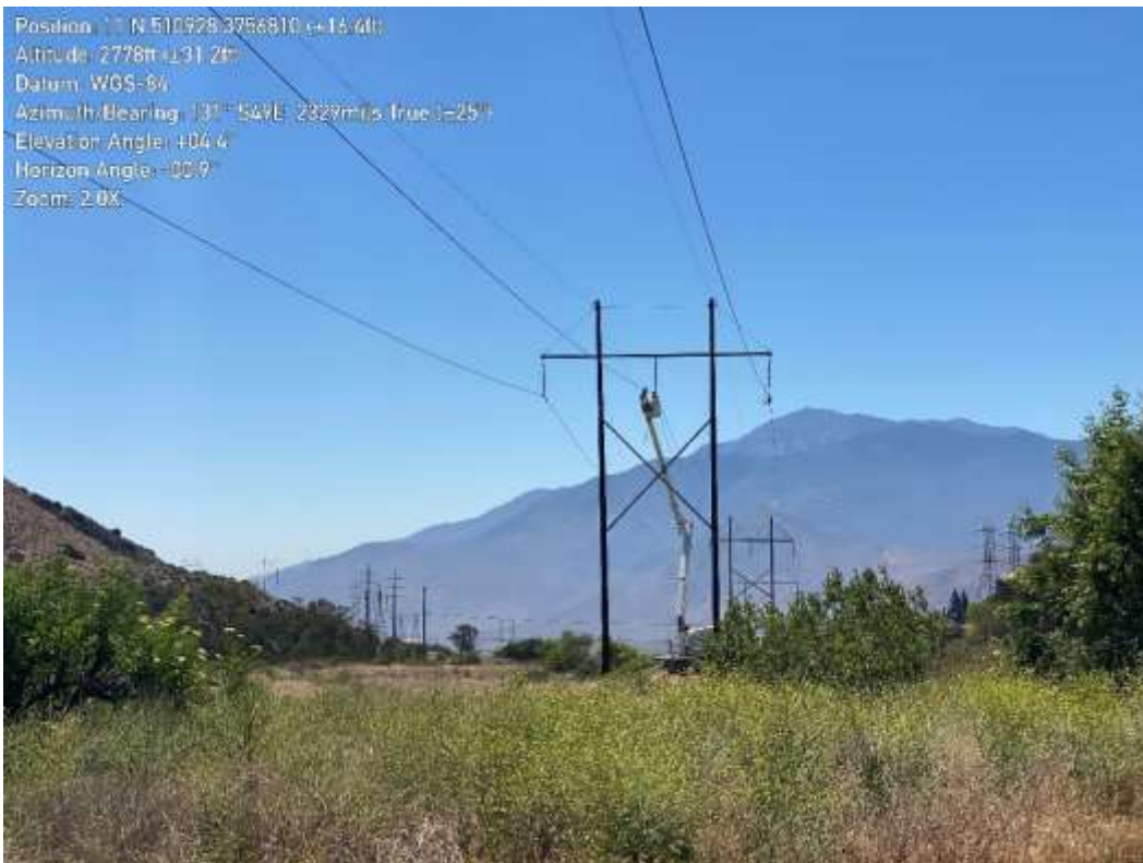
Photo 4 – Wire wreck-out activities at Construction Area PP123354, Segment 4 (June 4, 2021) (Photo courtesy of SCE).
