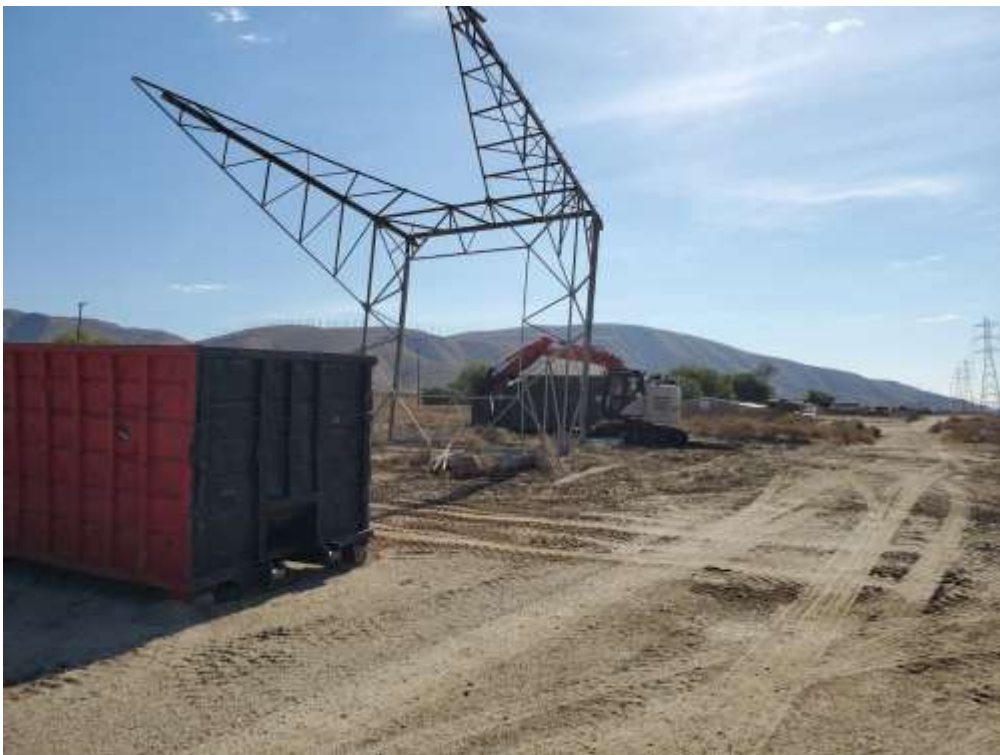
Photo 2 – Tower shearing at Construction Area 6N40, Segment 6 (July 7, 2021)
