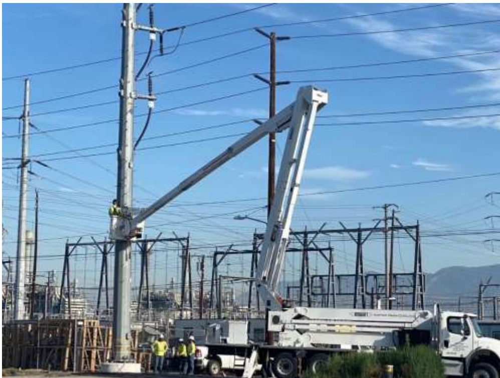
Photo 2 – Punch-list activities at Subtrans Pole 4696055E, Segment 1 (July 28, 2021) (Photo courtesy of SCE).
