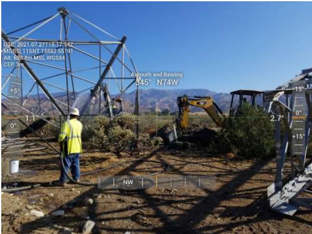
Photo 5 – Foundation wreck-out at Construction Area 5X24, Segment 5 (July 27, 2021) (Photo courtesy of SCE).
