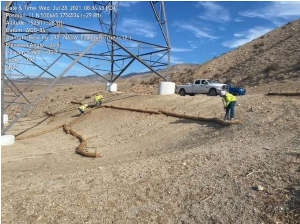
Photo 6 – BMP installation at Construction Area 6N32, Segment 6 (July 28, 2021) (Photo courtesy of SCE).
