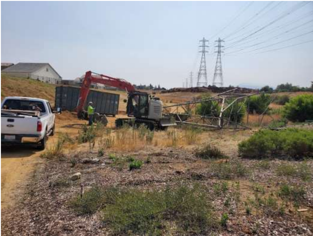
Photo 3 – Tower shearing at Construction Area PP123288, Segment 4 (August 17, 2021).
