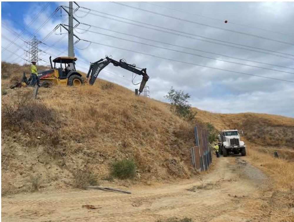
Photo 2 – Foundation wreck-out at Construction Area 2N01-WSS, Segment 2 (August 18, 2021) (Photo courtesy of SCE).
