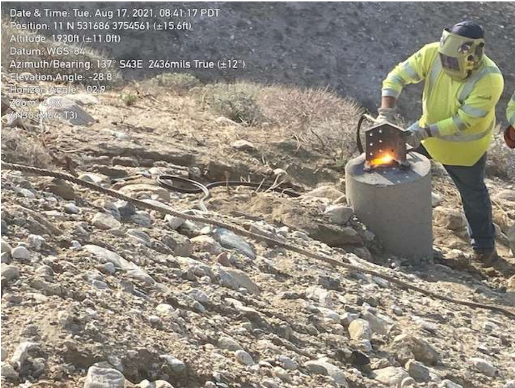
Photo 4 – Foundation wreck-out at Construction Area 6N30, Segment 6 (August 17, 2021) (Photo courtesy of SCE).
