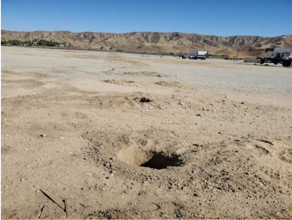
Photo 1 – Line of open steep-walled holes for fencing at the Poultry MY (September 15, 2021).
