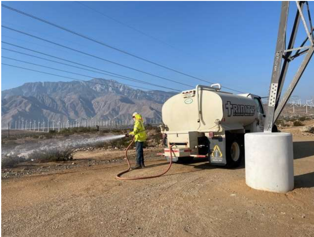
Photo 4 – Hydroseed watering at Construction Area 6X11, Segment 6 (September 27, 2021) (Photo courtesy of SCE).
