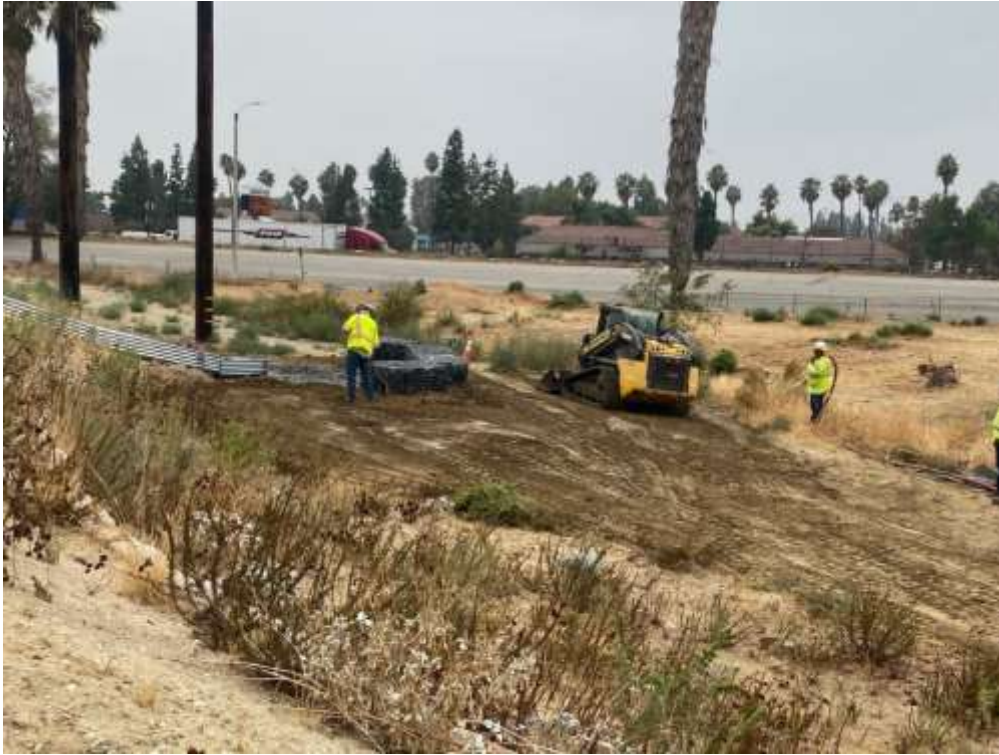
Photo 1 – Erosion repair at Construction Area 2N32, Segment 2 (September 21, 2021) (Photo courtesy of SCE).
