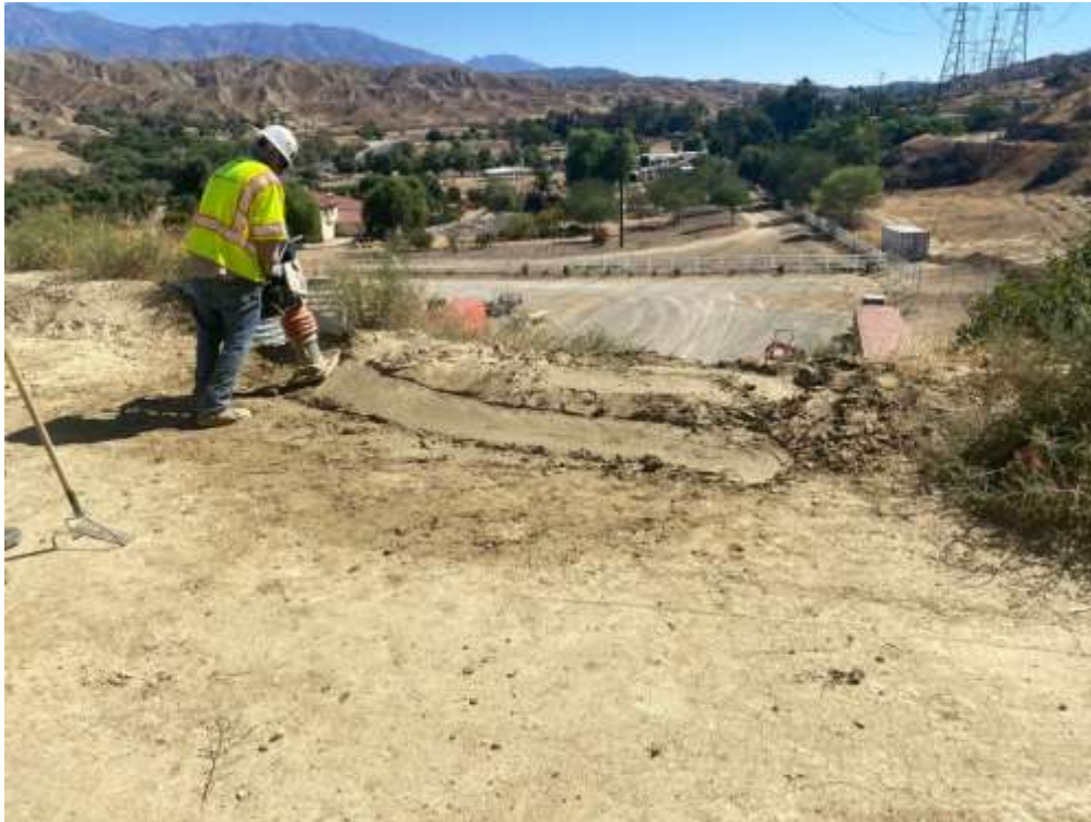
Photo 2 – Punch-list activities at Construction Area 3X28, Segment 3 (October 1, 2021) (Photo courtesy of SCE).
