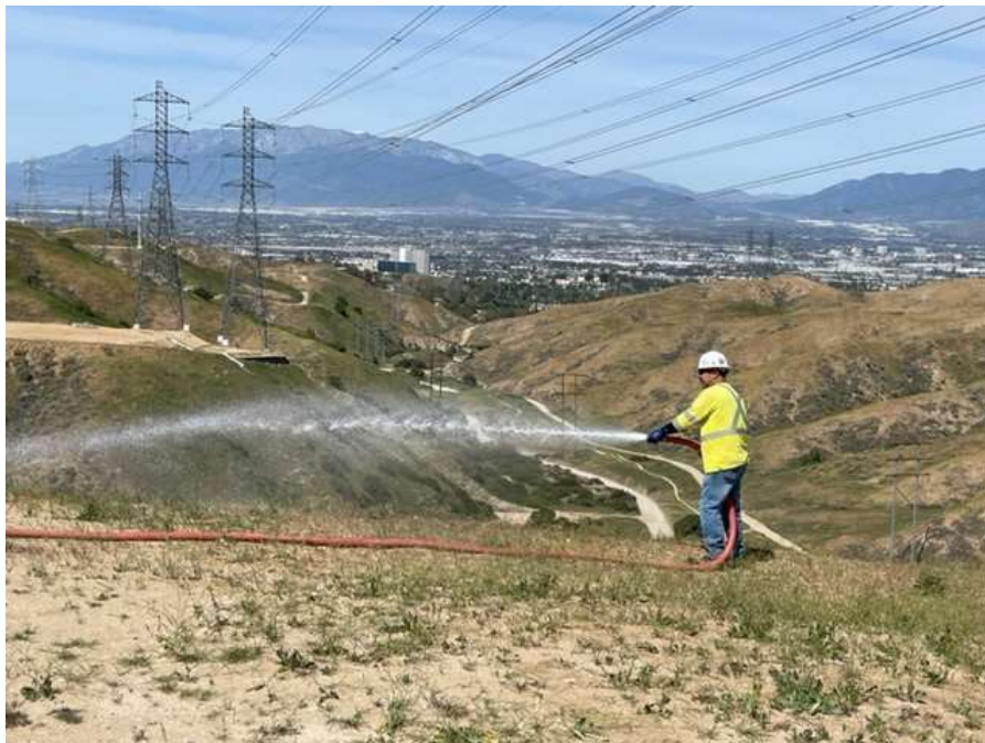
Photo 2 – Hydroseed watering at Construction Area 3X63, Segment 3 (March 21, 2022) (Photo courtesy of SCE).
