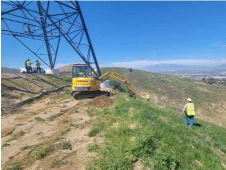
Photo 1 – Erosion Repair at Construction Area 2N12, Segment 2 (March 15, 2022) (Photo courtesy of SCE).
