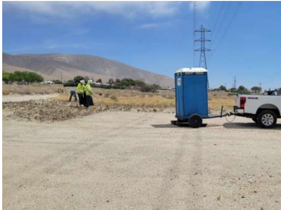
Photo 4 – Hand weeding at Construction Area 6N40, Segment 6 (April 11, 2022) (Photo courtesy of SCE).
