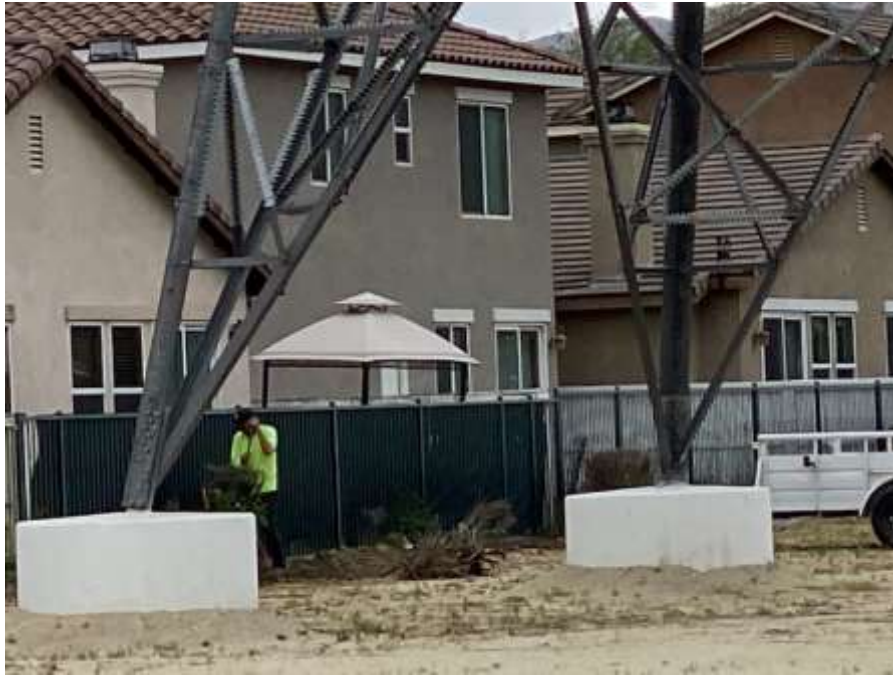
Photo 1 – Planter installation at Construction Area 1X13, Segment 1 (April 20, 2022) (Photo courtesy of SCE).
