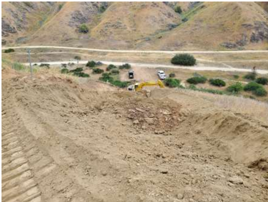
Photo 2 – Erosion repair at Construction Areas 3X64, WA-3-3N64-MPR-38, WA-3-3X64-MPR-53, and WA-3-3X64-MPR-54, Segment 3 (April 11, 2022).
