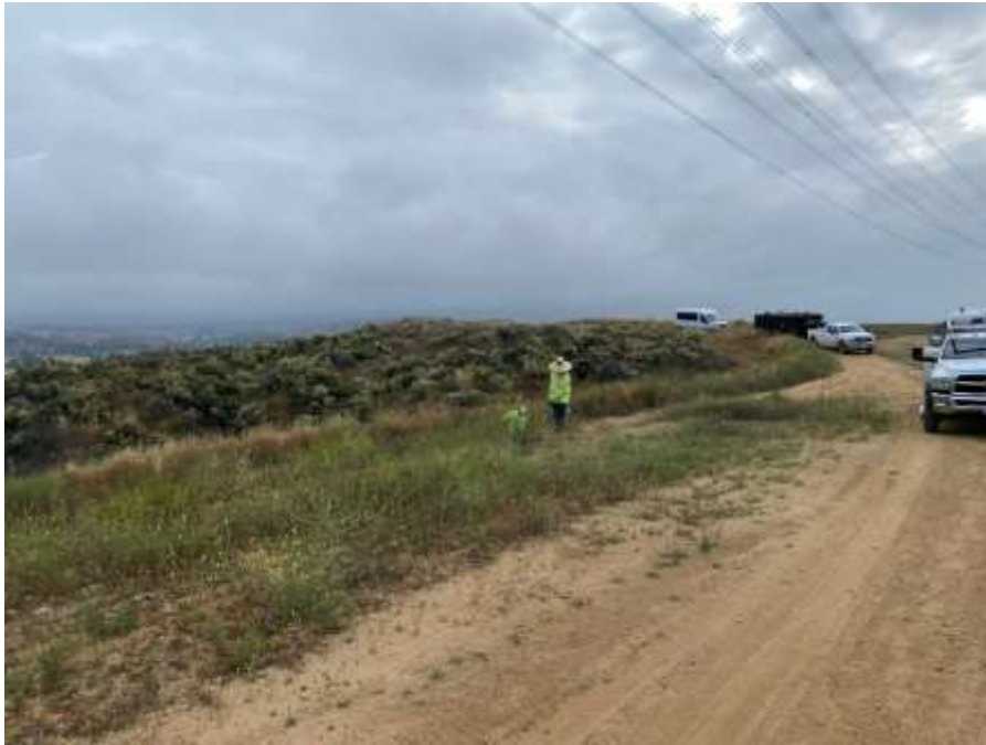
Photo 1 – Restoration site weeding at Construction Area 4X56, Segment 4 (May 31, 2023) (Photo courtesy of SCE).
