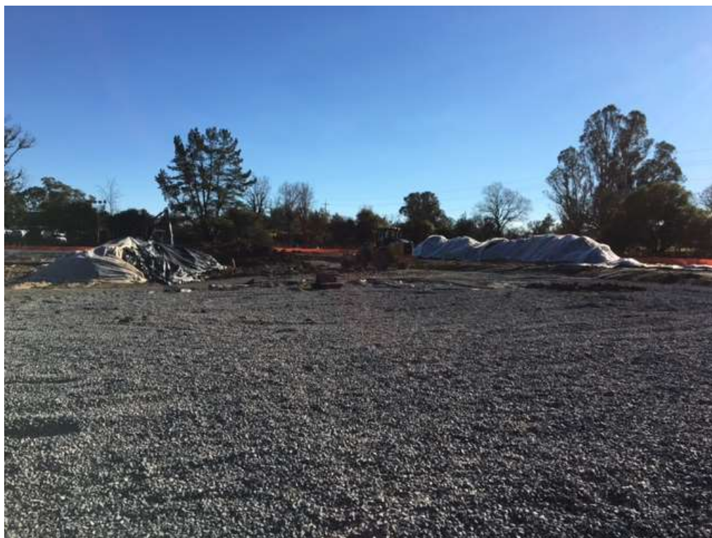
Figure 2 – Soil piles covered with plastic at the substation site – view south, January 5, 2017.
