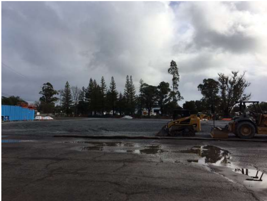
Figure 3 – Substation site after storm event – view south, January 11, 2017.
