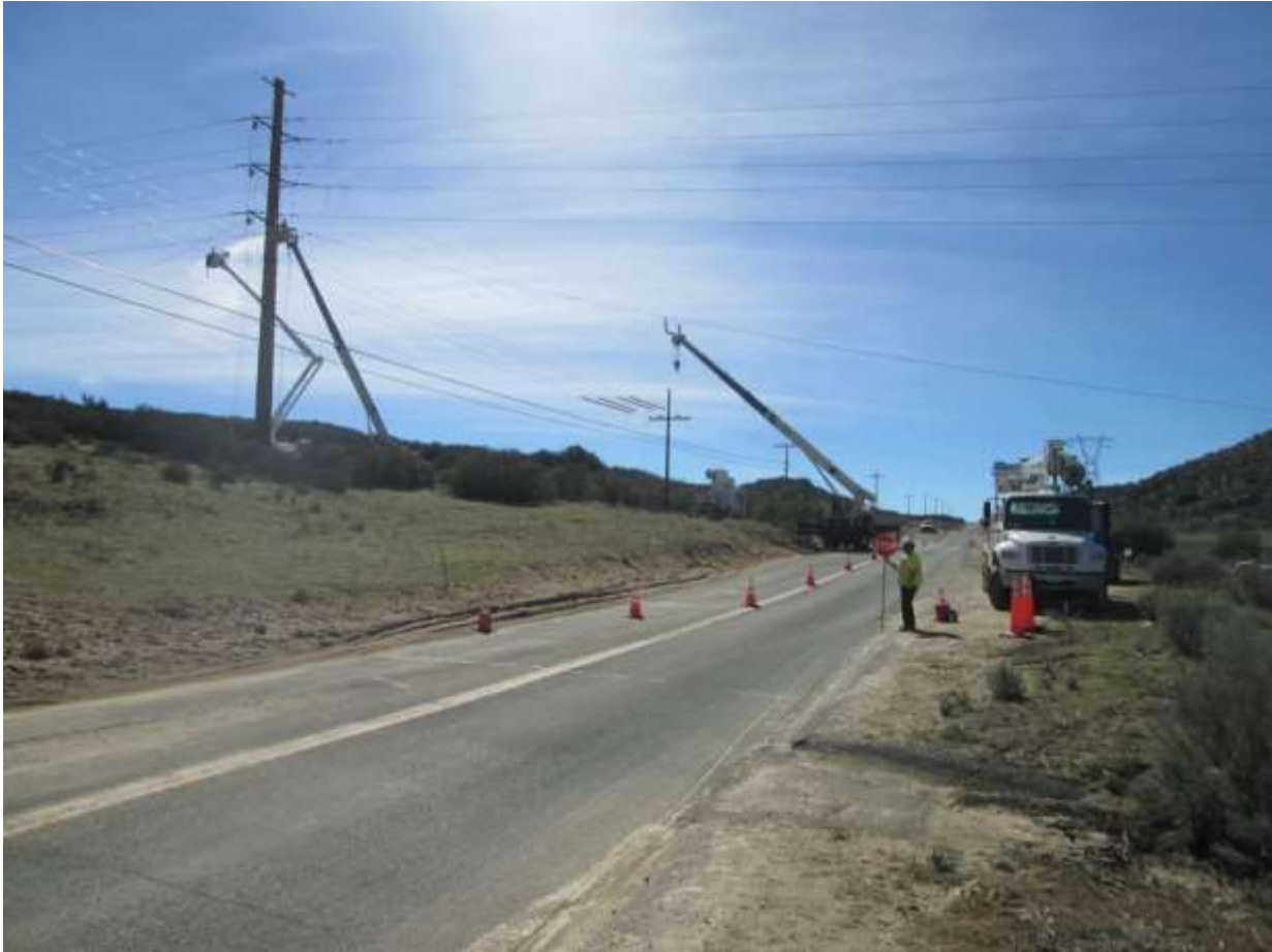
Photo 6: During wire stringing activities at Pole Z44173 and across La Posta Road (TL 629E), notification signage, cones, and flag persons were observed being utilized to direct traffic safely through the construction zone, where a lane was closed to stage a mobile guard structure unit.
