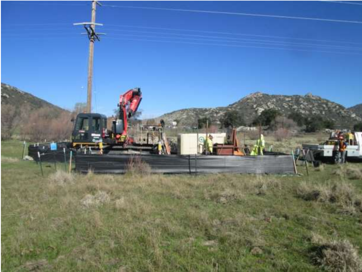
Photo 4: During micropile drilling at Pole Z40577 (TL 629E), Arroyo Toad protection measures were observed being implemented in accordance with the Streambed Alteration Agreement, and included the use of exclusionary fencing around the workspace perimeter and the presence of a qualified biological monitor.
