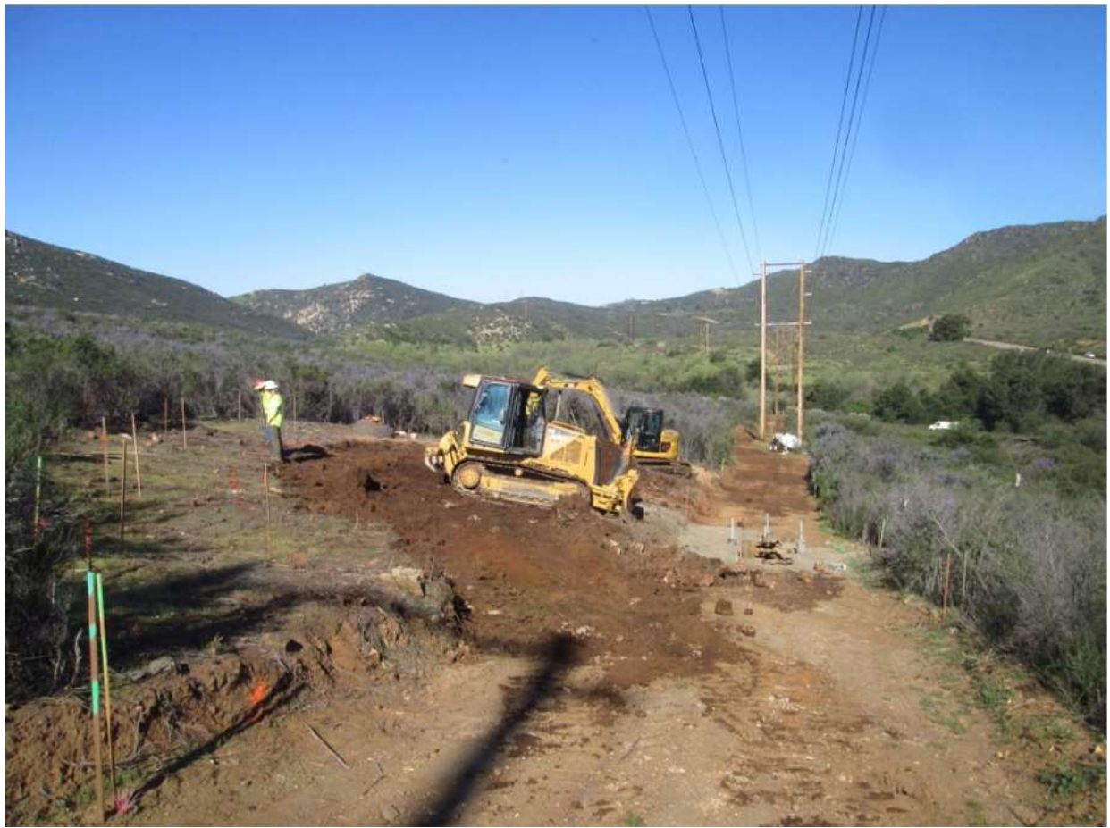
Photo 1: During access road widening at Z272867 (TL 625B), a grading crew was observed working within the delineated workspace in accordance with MM-BIO-1, and salvaging topsoil for future restoration use in accordance with MM-BIO-4.
