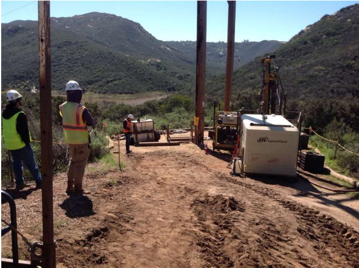
Photo 4: In accordance with MM CUL-1, cultural monitors were observed monitoring sites near ESAs along TL 625B.
