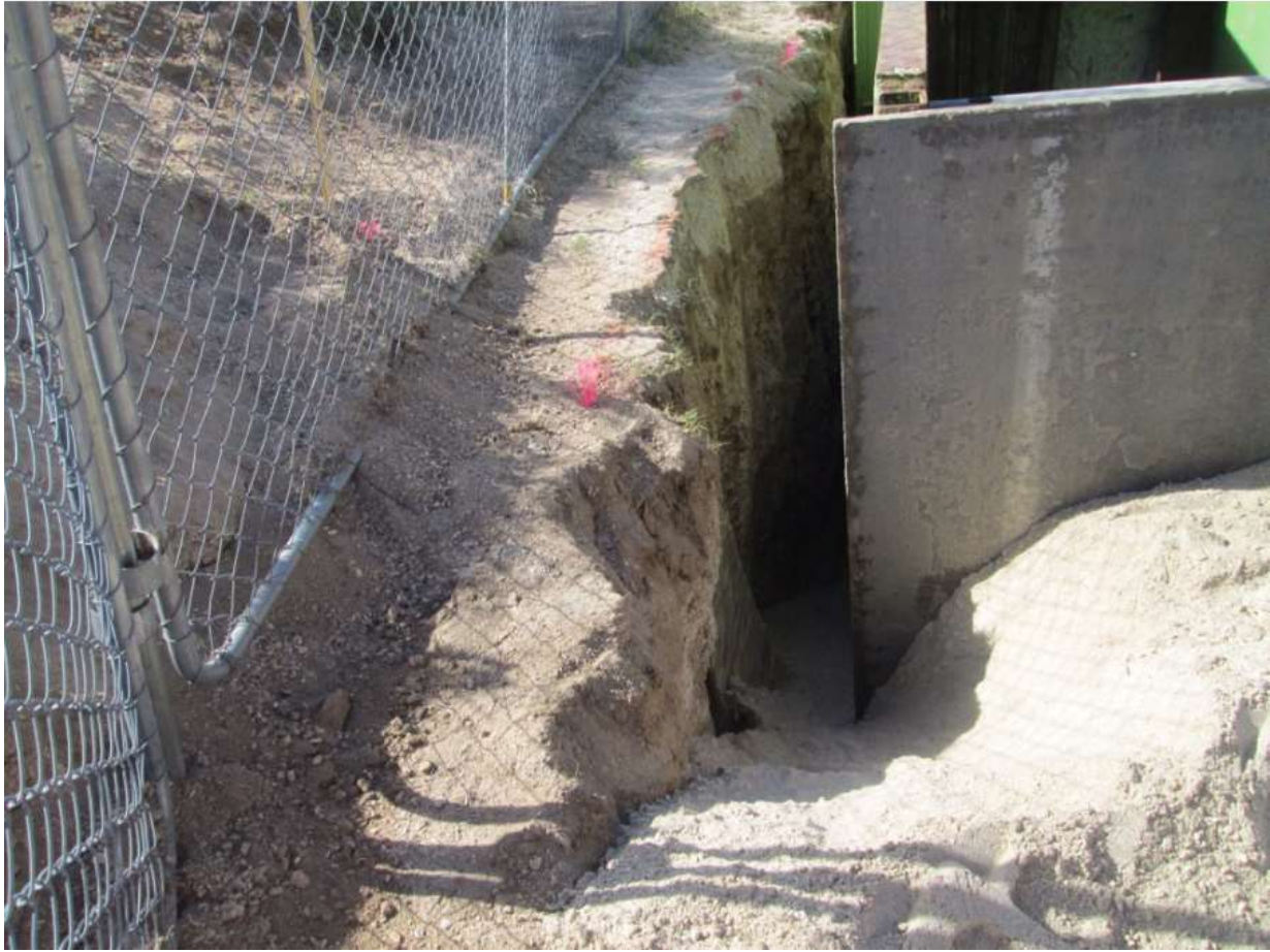
Photo 6: The bore pit (Crestwood Substation to Z100035, underground) had an earthen ramp constructed to prevent wildlife entrapment in accordance with MM BIO-23.
