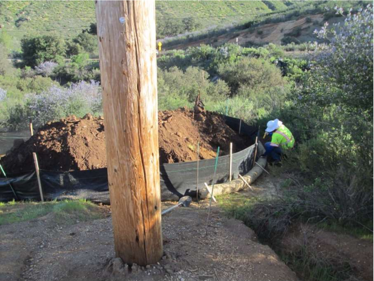
Photo 5: A construction worker observed installing fiber rolls (in addition to silt fencing) around the perimeter of a topsoil stockpile at Z272867 (TL 625B) in accordance with MM HYD-1 and MM BIO-4).
