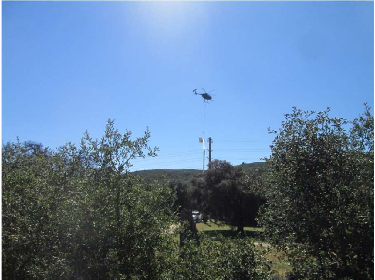
Photo 4: A construction crew was observed utilizing a helicopter to string sock line at Z40584 for fiber optic wire stringing between Z40572 to Z44182 (TL 629E).
