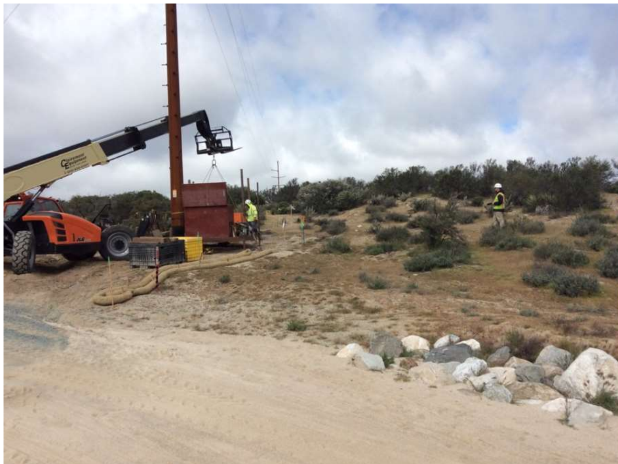
Photo 5: A qualified Avian Biologist was observed monitoring constructing activities adjacent to Pole Z44294 (TL 6931) near active nests in accordance with MM-BIO-28 in accordance with MM BIO-28 and the NBMP.
