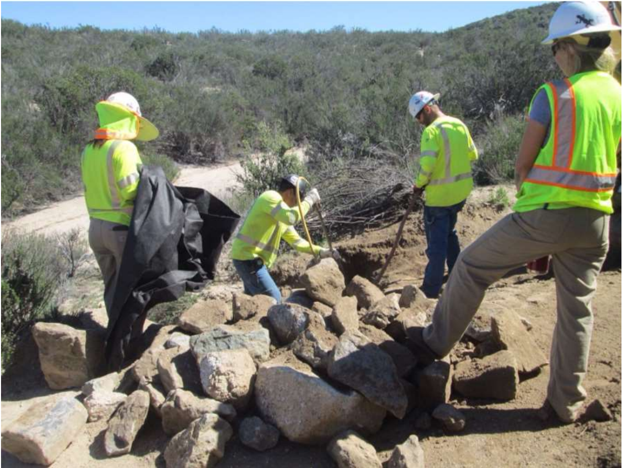
Photo 6: Geo Pacific Services crew observed performing energy dissipater maintenance along the access road between Z44173 and Z44175 (TL 629E) in accordance with MM-HYD-1.
