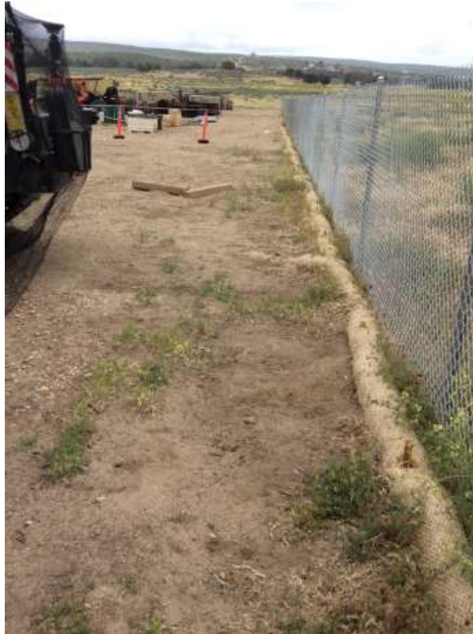
Photo 3: Erosion control BMPs such as fiber rolls were observed around the perimeter of Live Oak Springs Staging Area in accordance with the project SWPPP (MM HYD-1, MM BIO-7, and APM HYD-09).
