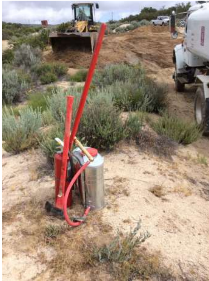
Photo 4: During grading of Stringing Site 21 (TL 6931), a set of fire tools was readily available within 50 feet of activity in accordance with the CFPPP (MM FF-1), APM HAZ-01 and APM HAZ-04.
