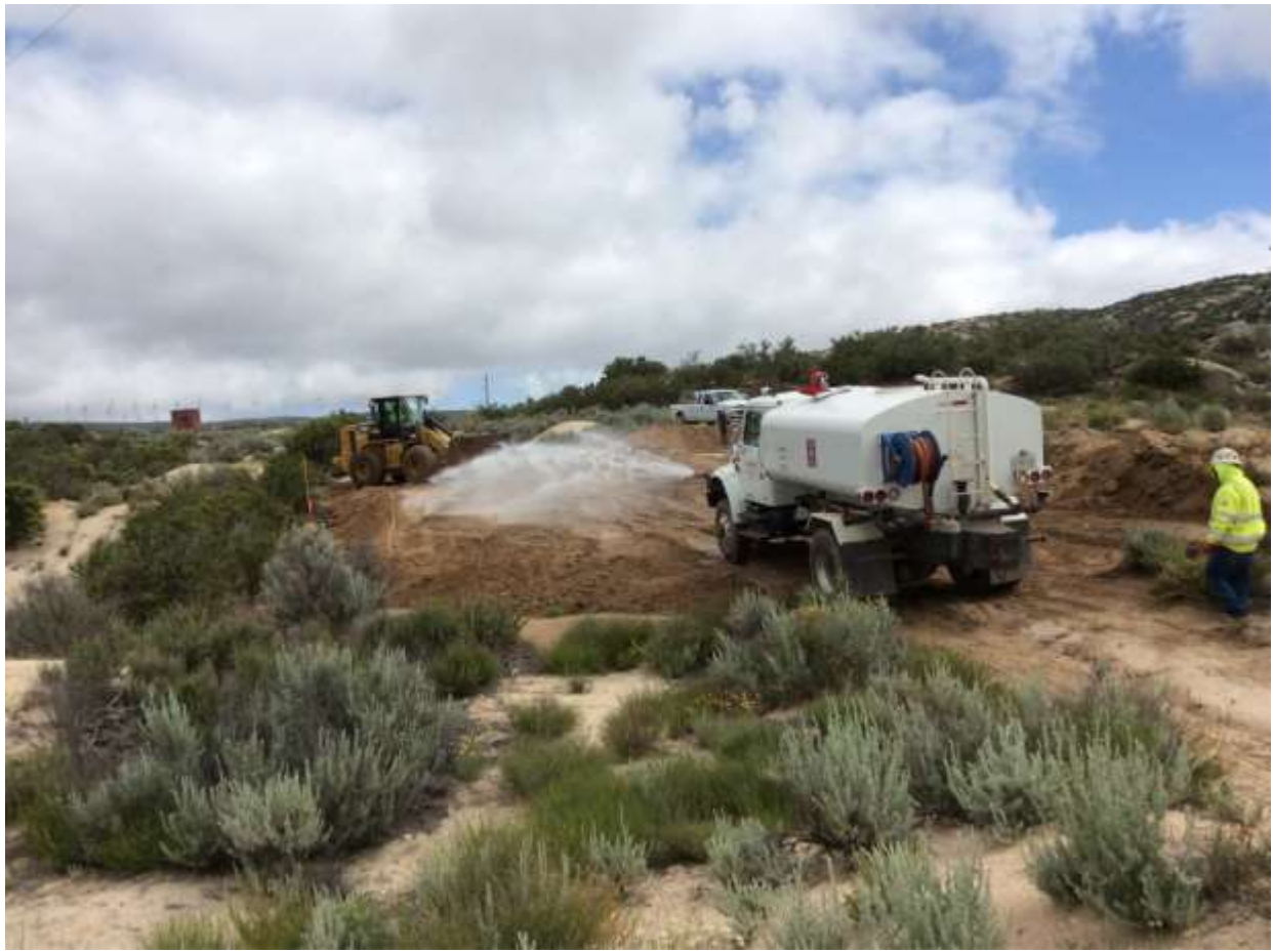
Photo 1: During grading of Stringing Site 21 (TL 6931), water was applied to prevent dust emissions in accordance with APM AIR-02.
