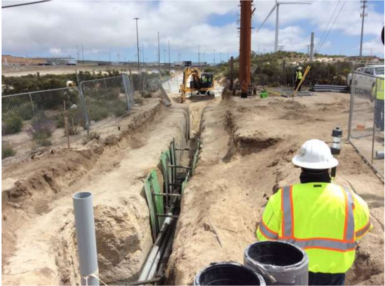
Photo 6: During trenching activities associated with the installation of underground utilities near Crestwood Substation (TL 629E), all work was observed being conducted within the delineated work limits in accordance with MM BIO-1, and a Native American monitor was present in accordance with MM CUL-1.
